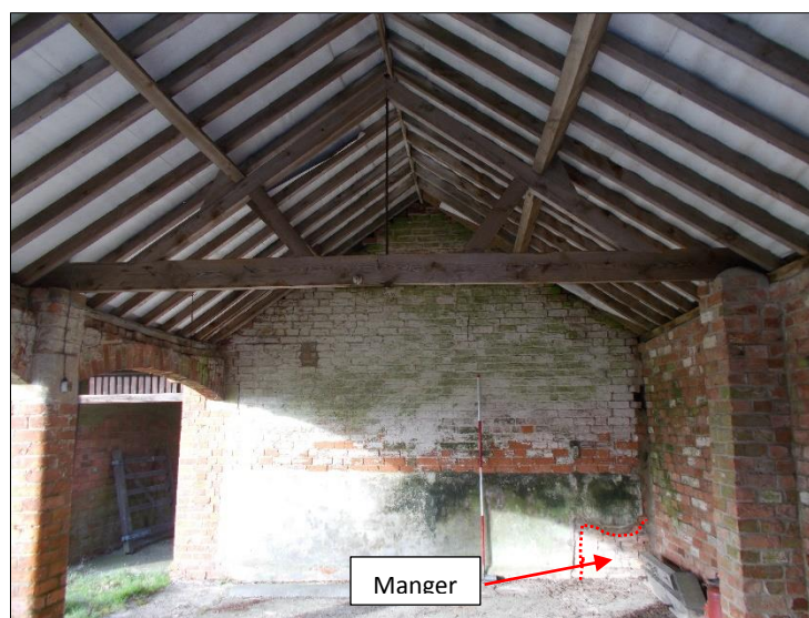
Fig 27: Room G6: The former livestock hovel, showing scar of former manger (red dotted line) and roof truss. Looking west. 2m scale rod.
