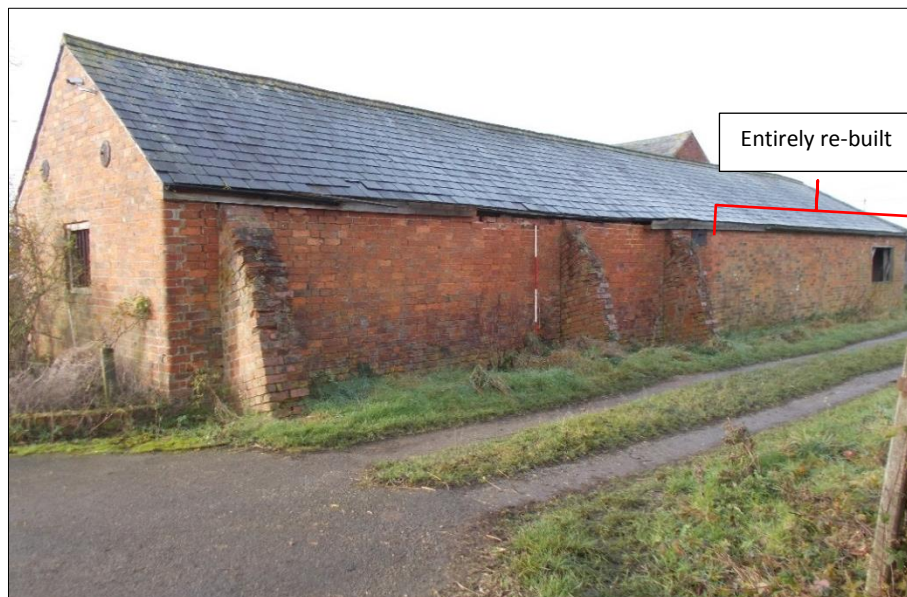
Fig 17: The north elevation of the eastern range, looking south-west. 2m scale rod.
