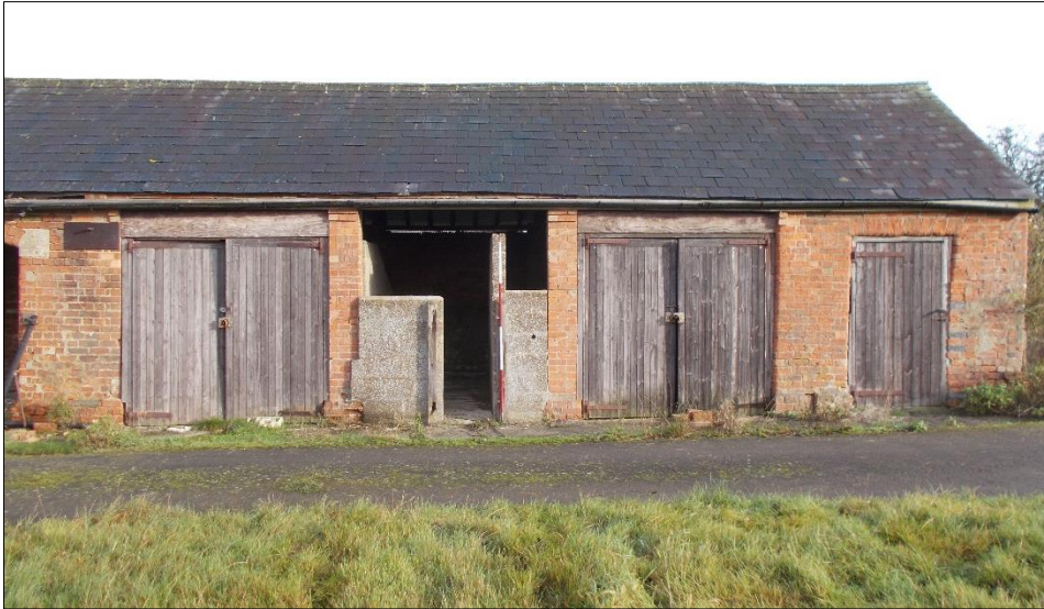
Fig 15: The south elevation of the eastern end of the eastern range, looking north. 2m scale rod.
