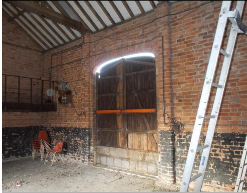
Fig 25: Room G4, the store barn showing the inner surface of the cart door, looking south-west.
