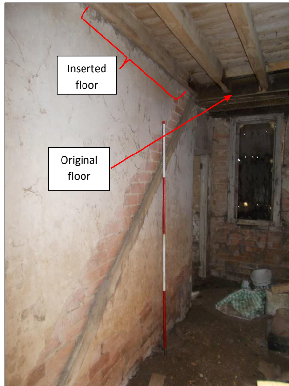
Fig 19: The former stairwell, looking west. Note timber string batten to left. 2m scale rod.
