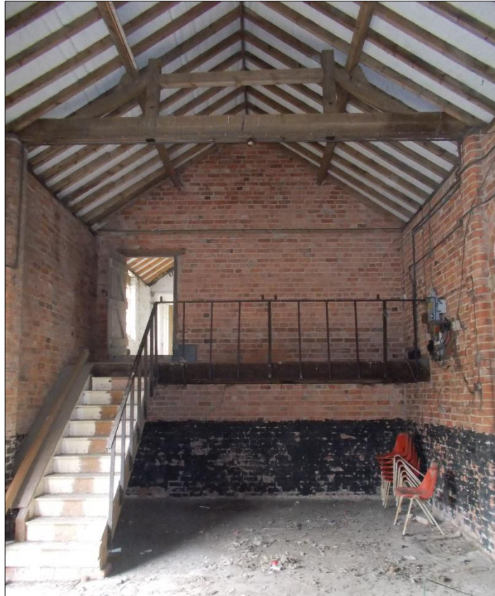
Fig 24: Room G4, looking south showing south wall with secondary stairs, balcony and doorway. Note also roof truss configuration and buttressing.
