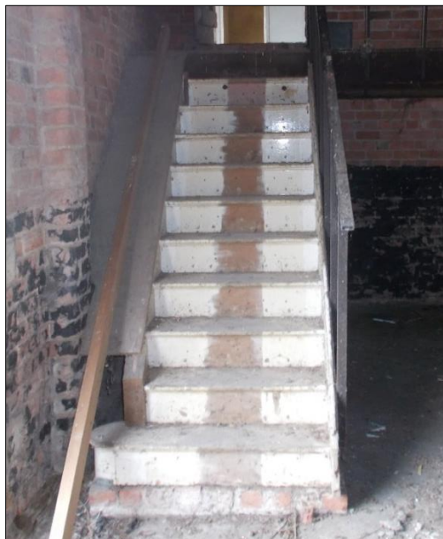
Fig 26: The inserted staircase in G4, looking south. Note rounded and projecting lower tread (left) and the paint scheme for a stair runner.
