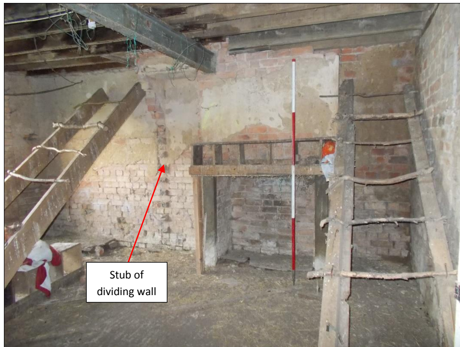
Fig 20: Room G3, looking north showing former fireplace and dividing wall. 2m scale rod.
