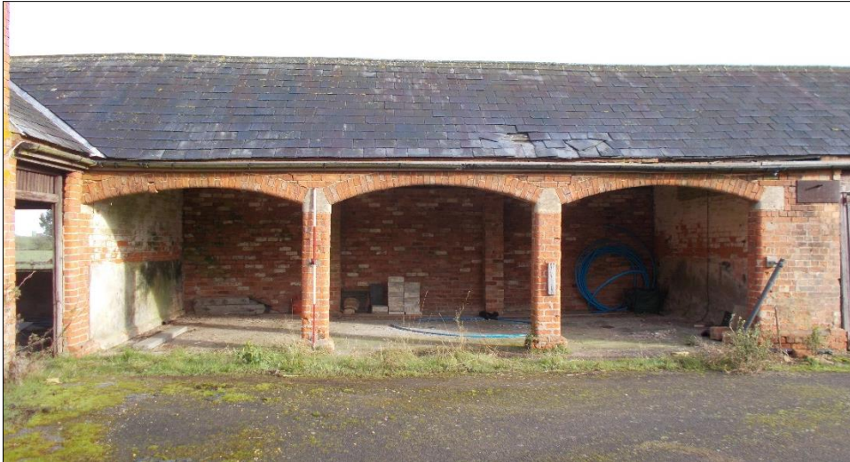
Fig 13: The three-arched western section of the eastern range, looking north. 2m scale rod.
