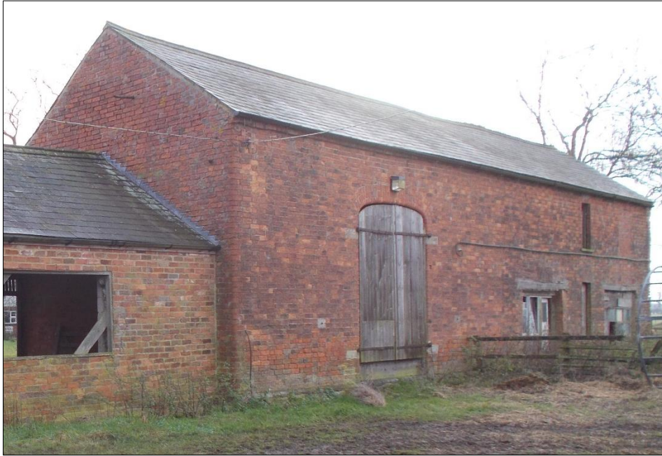
Fig 5: The north gable (left) and west elevation of the western range, looking south-east.
