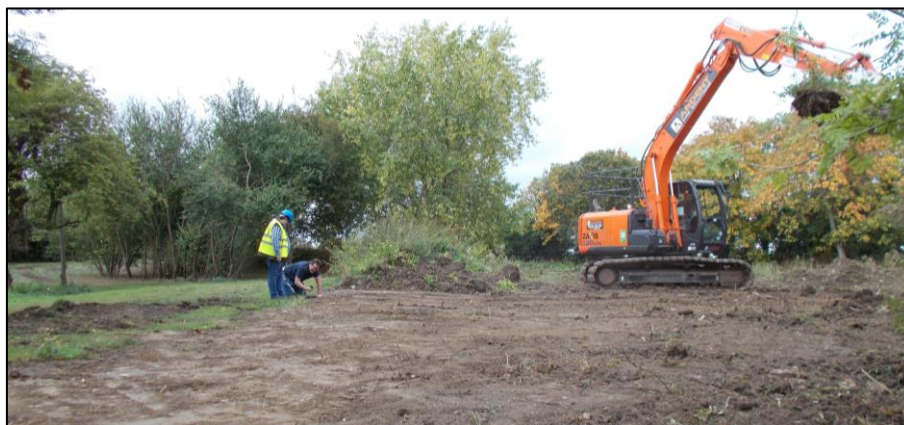
Fig 11: Spreading the bund, here about 1.2m high. Note the newly-reunified ground levels to either side.
