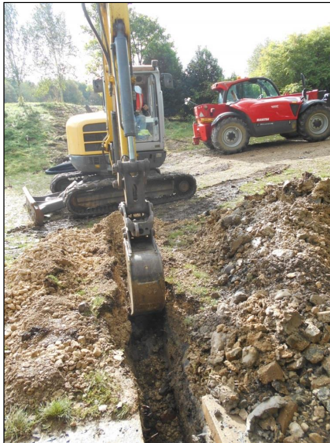
Fig 6: Commencement of the pipeline at the manor service shed, looking north. In the background the escarpment which marks the north edge of the cricket field.
