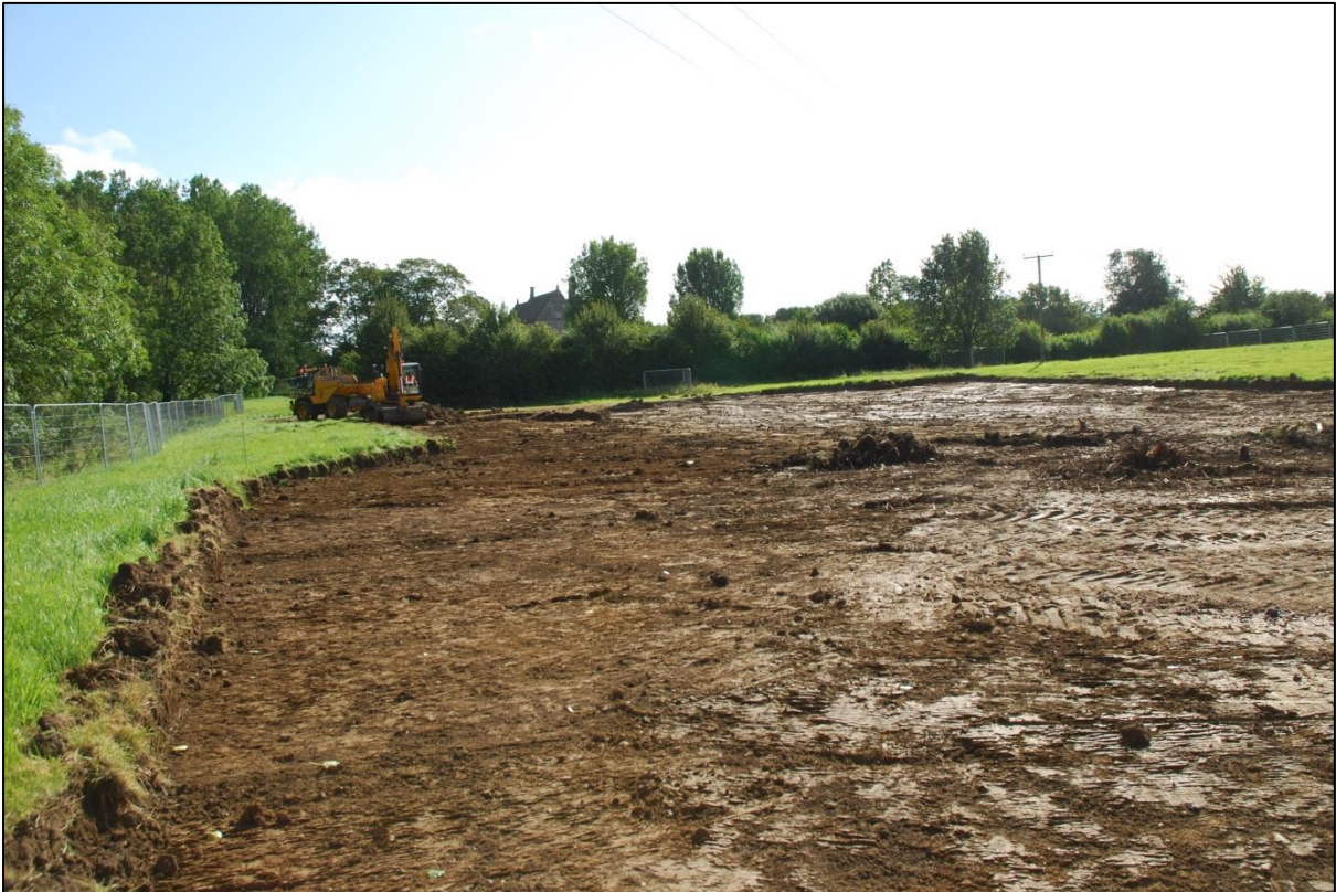
Fig 3: New Car Park area, stripped of topsoil and subsoil, looking east. Manor House in the distance.
