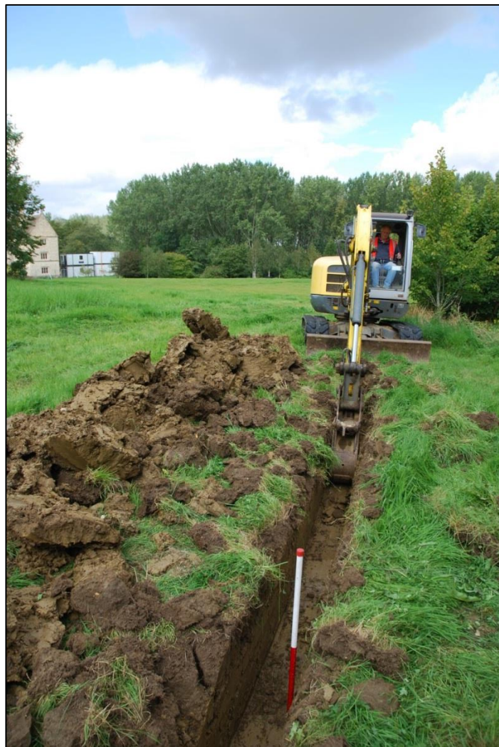
Fig 7: Machining south of the cricket field and swinging out around trees, looking north-west with manor in the background; Scale 1m
