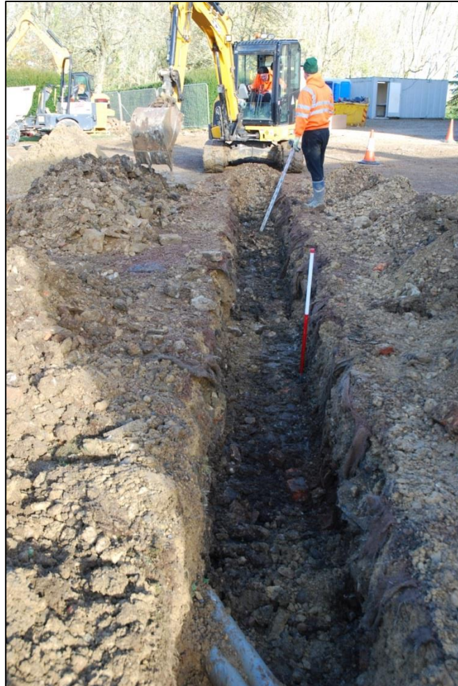
Fig 5: View along the courtyard service trench (southern third), looking north-east; scale 1m. The light grey plastic ducts in the foreground were laid for BT -WAN enhancement in 2018 (see Soden 2018)
