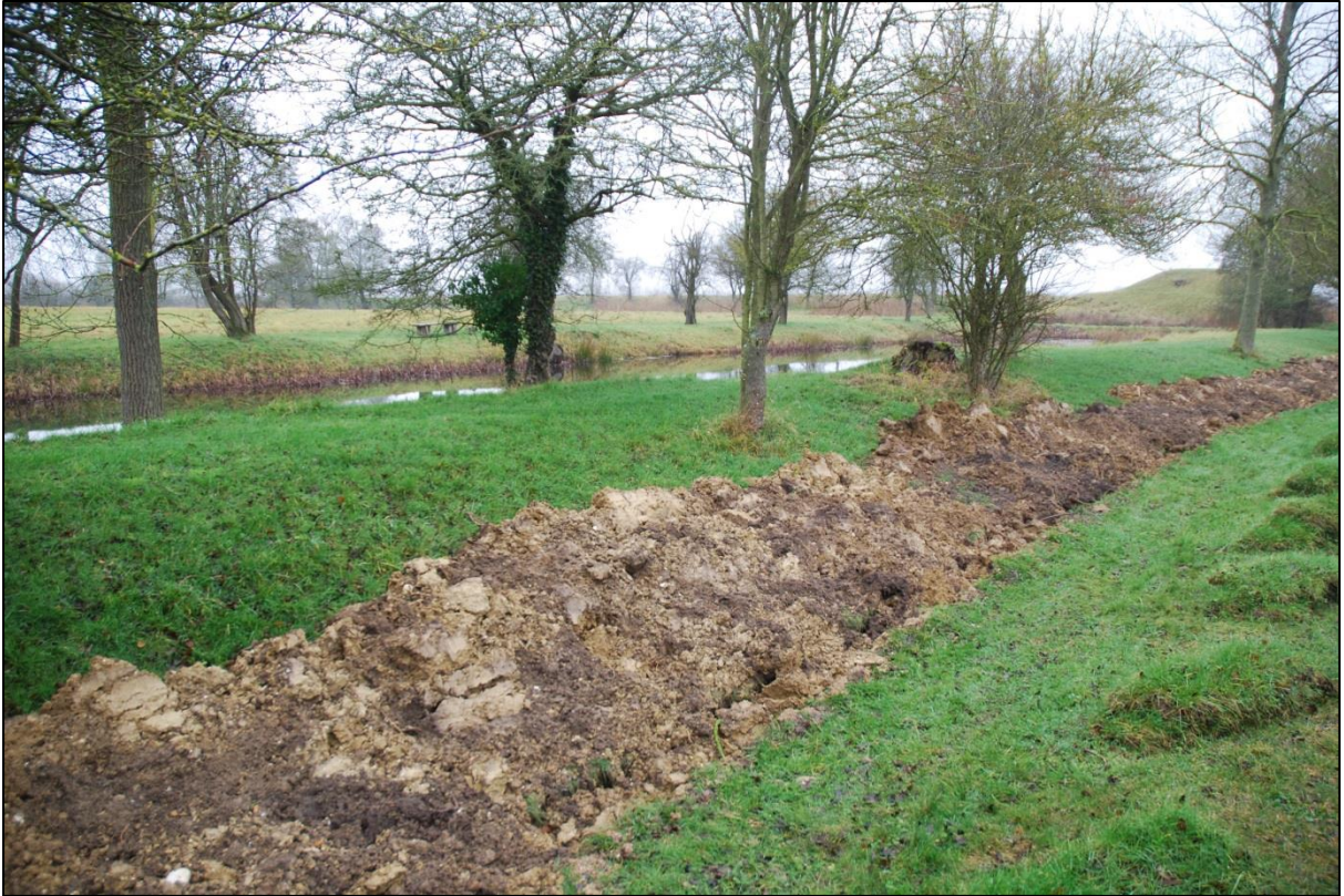
Fig 10: Alongside the moat. Here the trench flooded so it was quickly backfilled.
