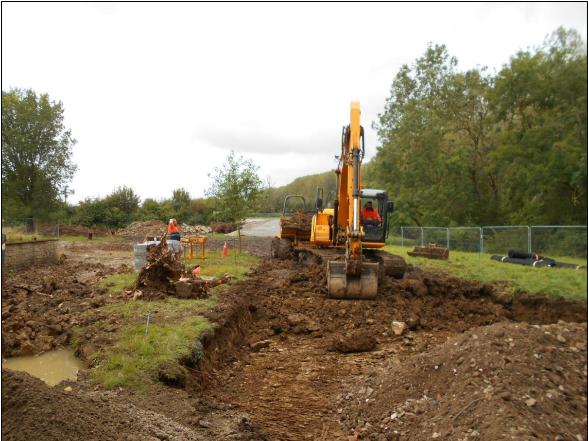
Fig 4: Digging out and stoning-up the access road to the car park, looking west
