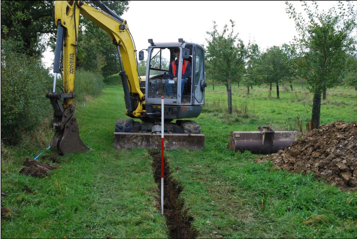
Fig 9: Machining along the orchard's eastern boundary, looking south. The trench here was about 1.1m deep. Scale 2m in 0.5m graduations.
