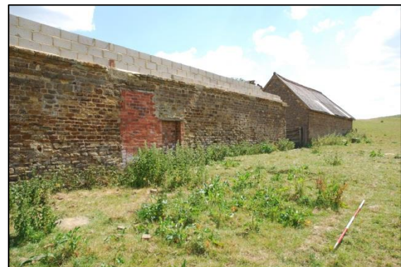
Fig 22: The south wall exterior. The two blocked door-heights probably relate to the original and a heightened wall. The 2m scale lies along surviving brick foundations of a demolished building.
