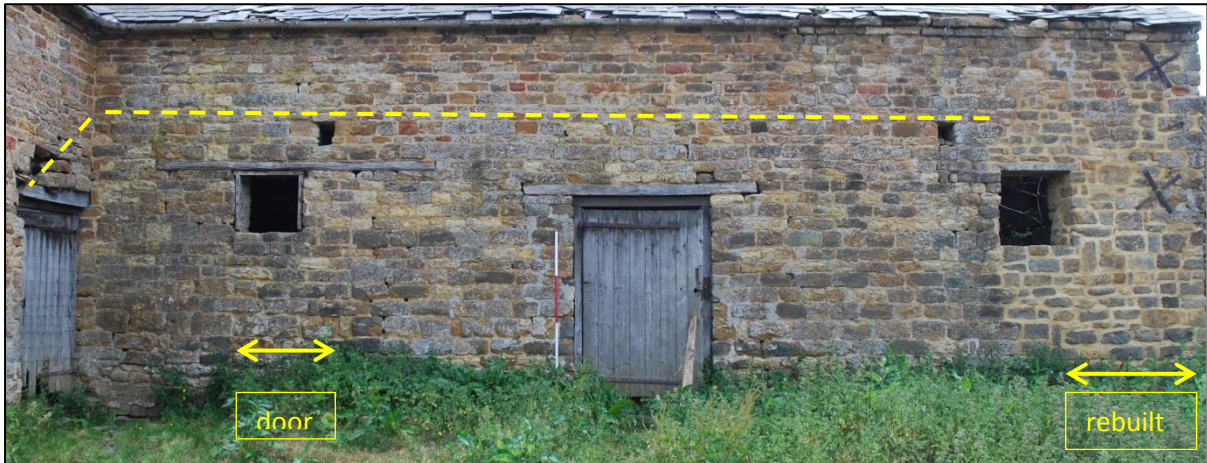
Fig 16: The farmyard elevation of the stable/cowhouse. The original door blocking and row of blocked joist sockets indicated; scale 2m
