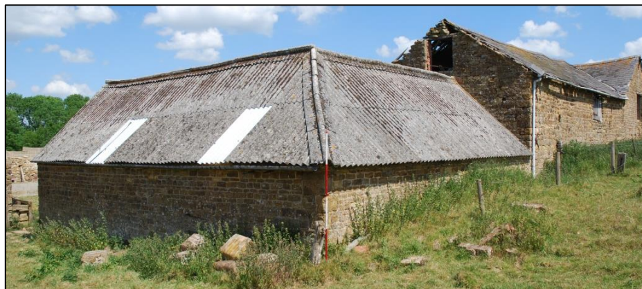
Fig 20: The cow-house exterior. Note the original pitching door above the stable which was made into a window when it became inaccessible; scale 2m
