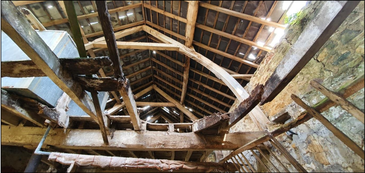
Fig 14: View of the southernmost Upper Cruck truss from the south end of the stable. Note the water tank and a sling-brace visible just above the wall. Unusually, the photo was taken with extreme wide angle on a phone-camera for coverage given the inaccessibility of the subject and to maximise the view of the crucks.
