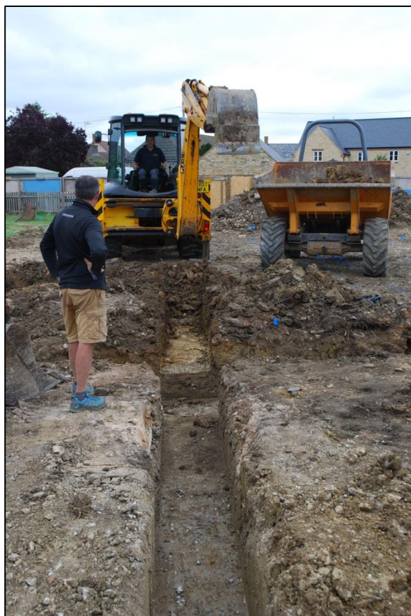
Fig 3: View of the foundation-digging looking east, uncovering a concrete foundation slab at depth
