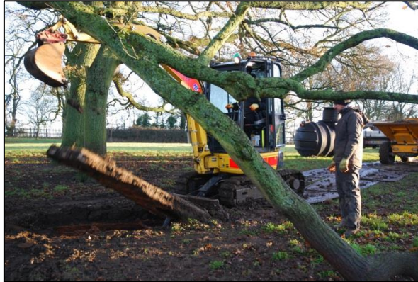
Fig 4: Breaking the old septic tank, here the reinforced concrete lid. In the background stands the new tank
