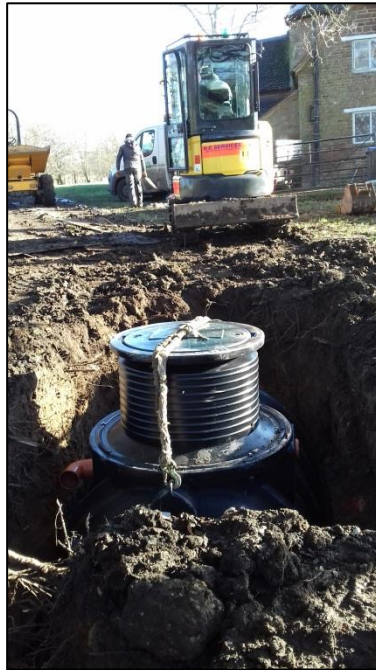
Fig 5: The hole for the new tank complete, with new tank in situ
