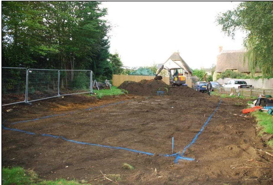
Fig 3: View across the site stripped of turf and most topsoil, looking west towards Rookery Cottage, 10 Duck End. The ring-foundation trench is marked out in blue and the tail of the terrace-bank is visible at left
