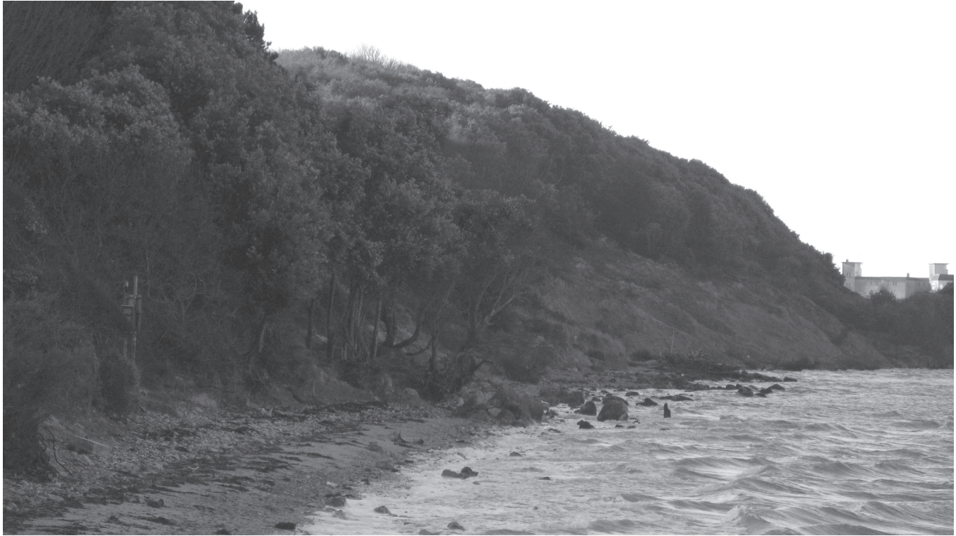
Figure 10.2 Rotational sliding is visible along the cliff at Fort Victoria Country Park, on the north-west coast of the Isle of Wight. The retreating cliff is 1.3km from Hurst Castle (Jan Gillespie)
