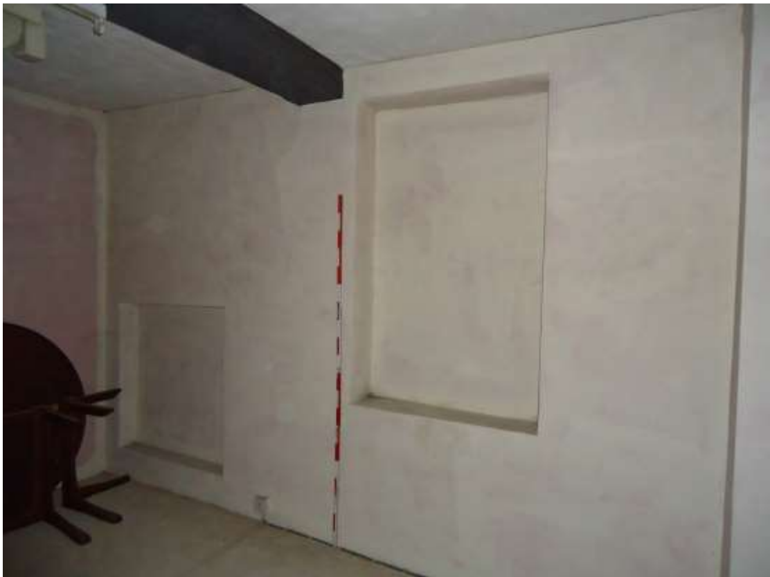
Plate 12; detail within the north corner at first floor level of front range.
