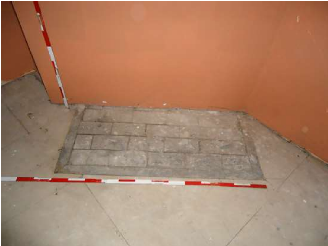
Plate 14; remains of second floor fireplace in the west corner of the rear range.
