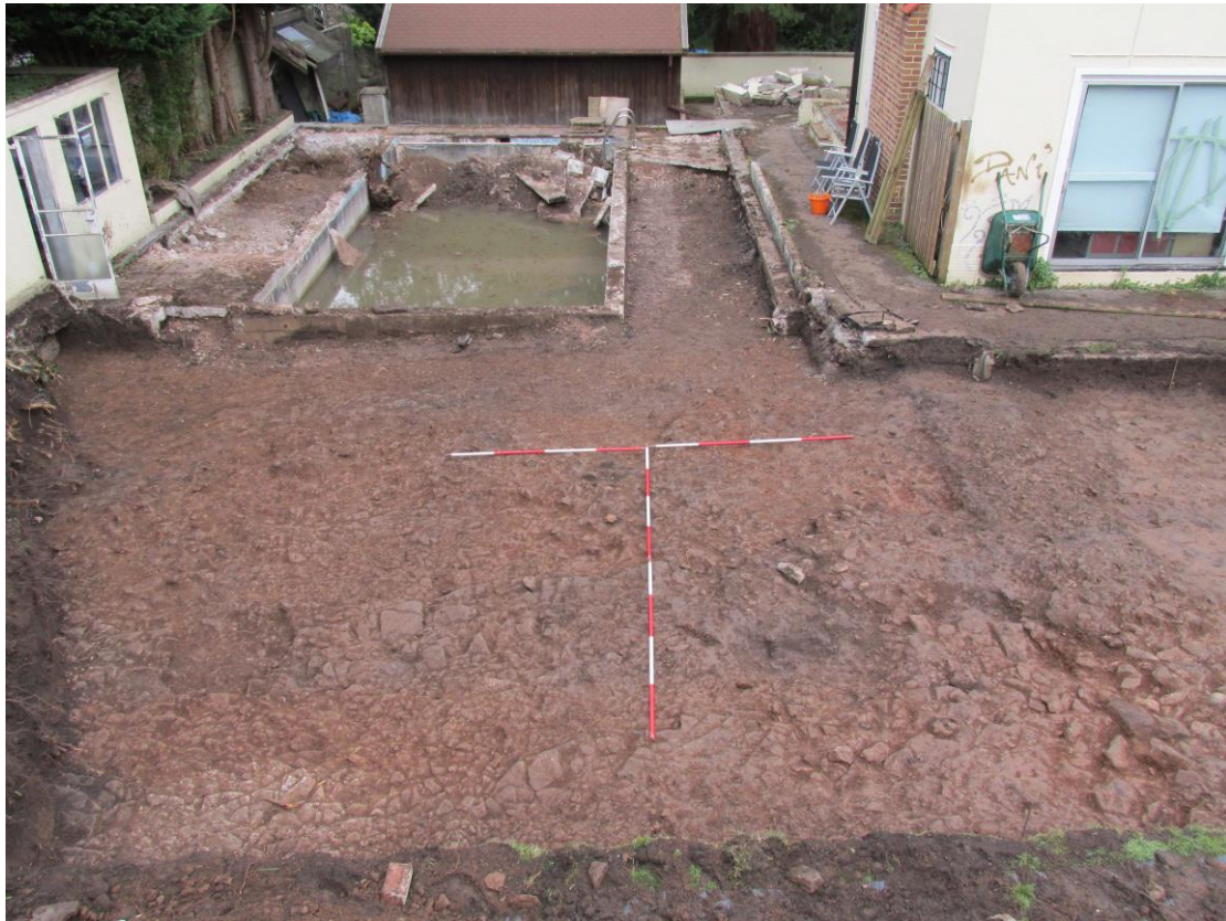
Plate 13; excavation area; view to the north-west, swimming pool and house (area of subsequent watching brief) in the background
