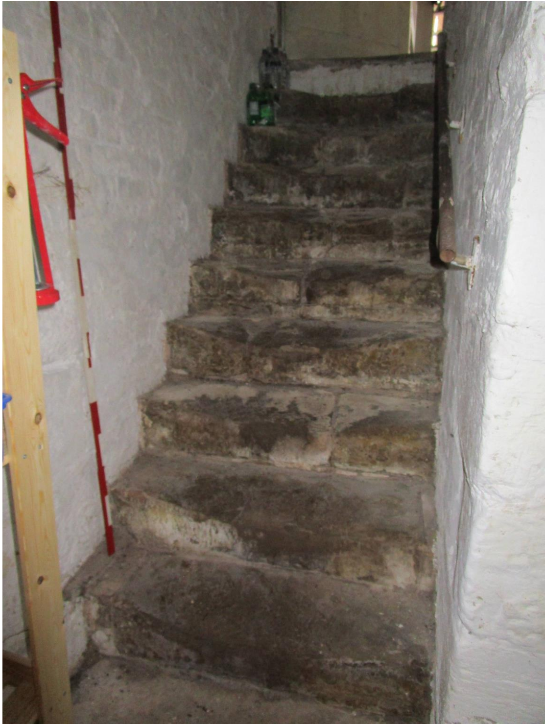
Plate 8; heavily worn steps to cellar.
