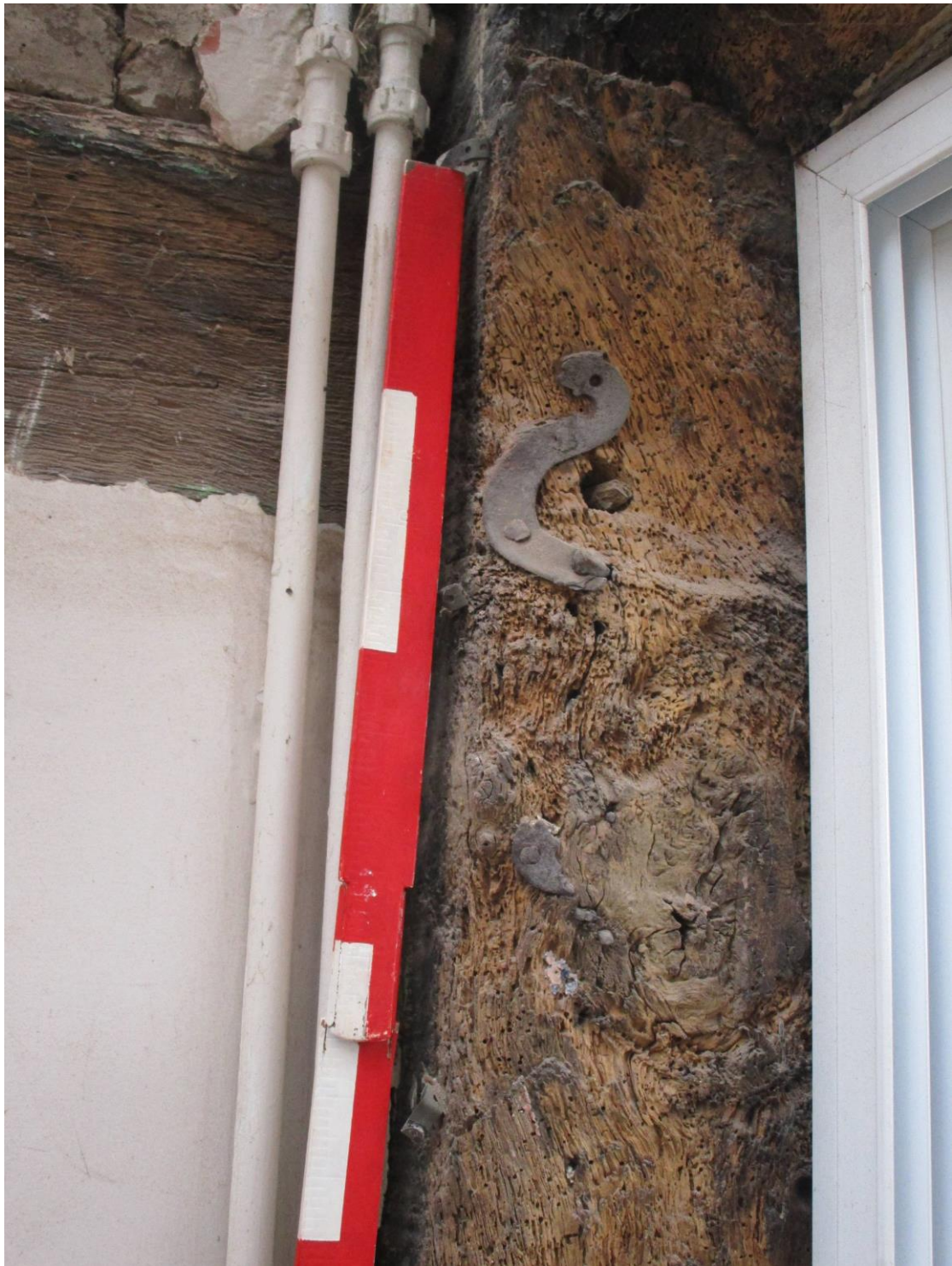
Plate 26; remains of cockscomb hinge (north-bay west-wall).
