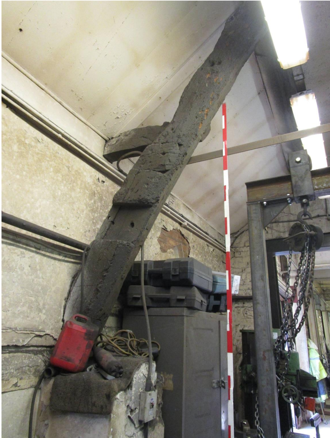
Plate 15; One of a pair of cruck-blades in single storey annexe to mill
