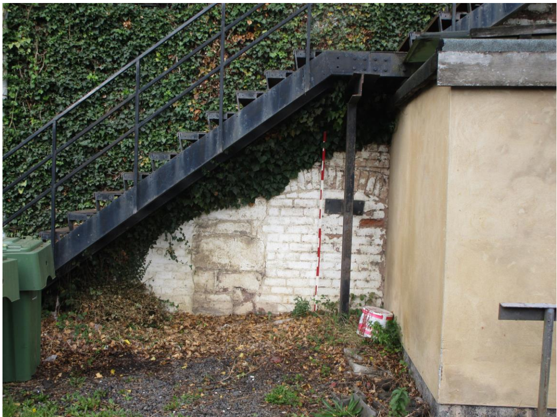
Plate 7; Blocked opening in front wall
