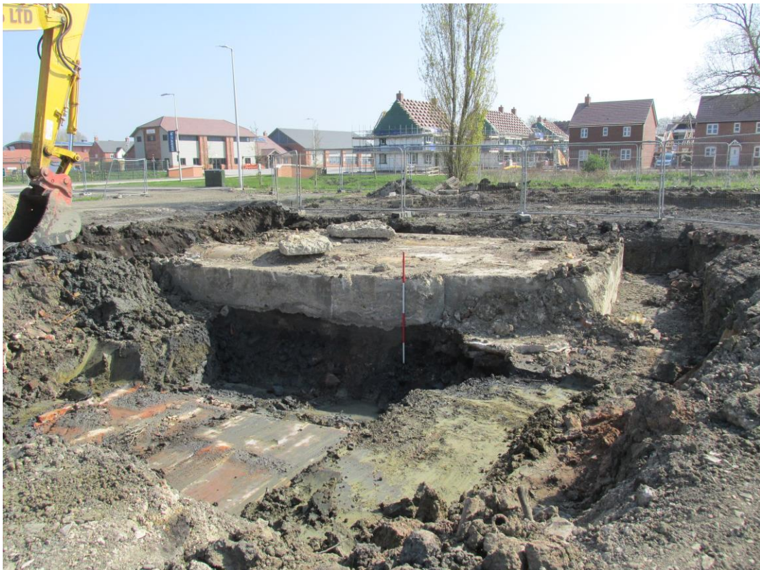
Plate 16; fuel storage tank
