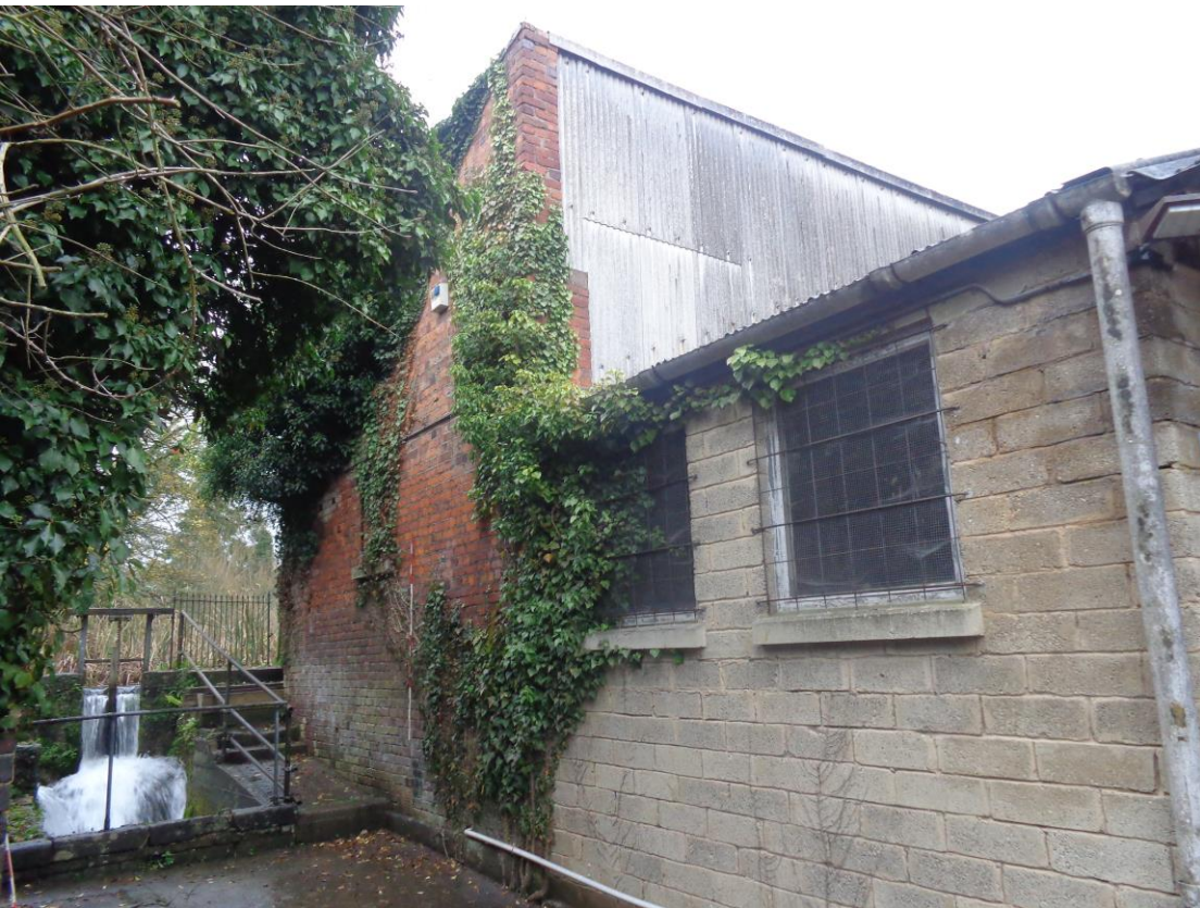
Plate 47; Building 10 from south-west showing blocked window
