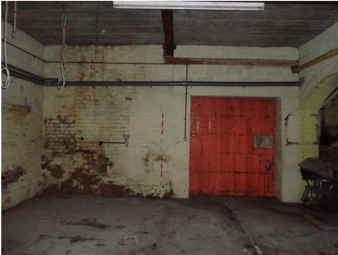
Plate 30; West end of former yard showing blocked opening (?for machine-belt) at north end of building 8
