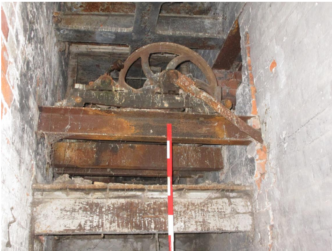
Plate 15; Stair-tower; remains of hoist mechanism and fire-damaged floor
