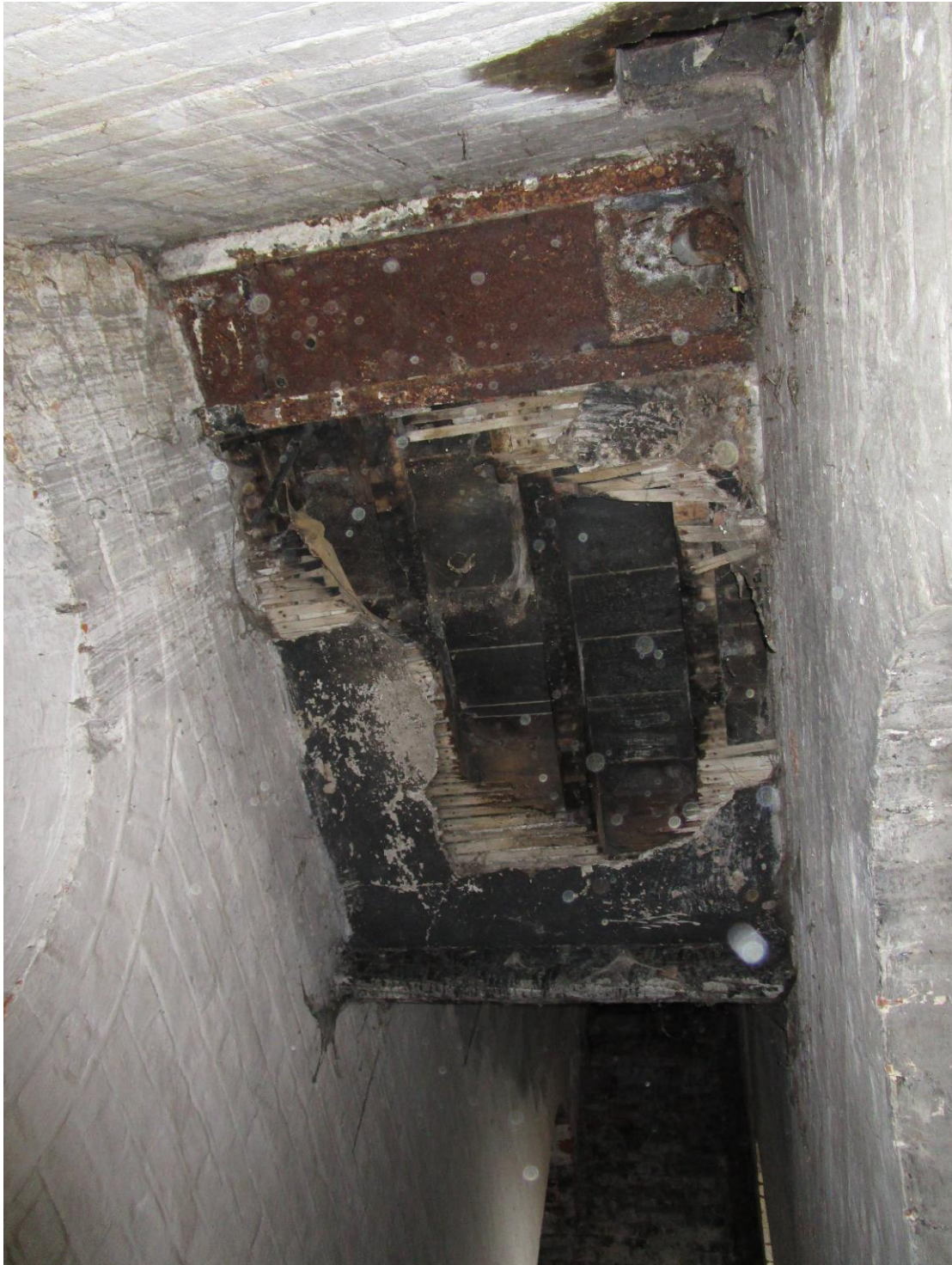
Plate 17; Stair-tower; underside of fire-damage floor
