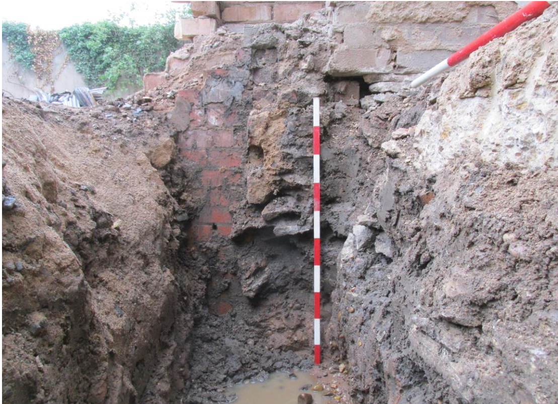
Plate 4; trench 1d, east end showing context (Lias stone wall) 112, from the west
