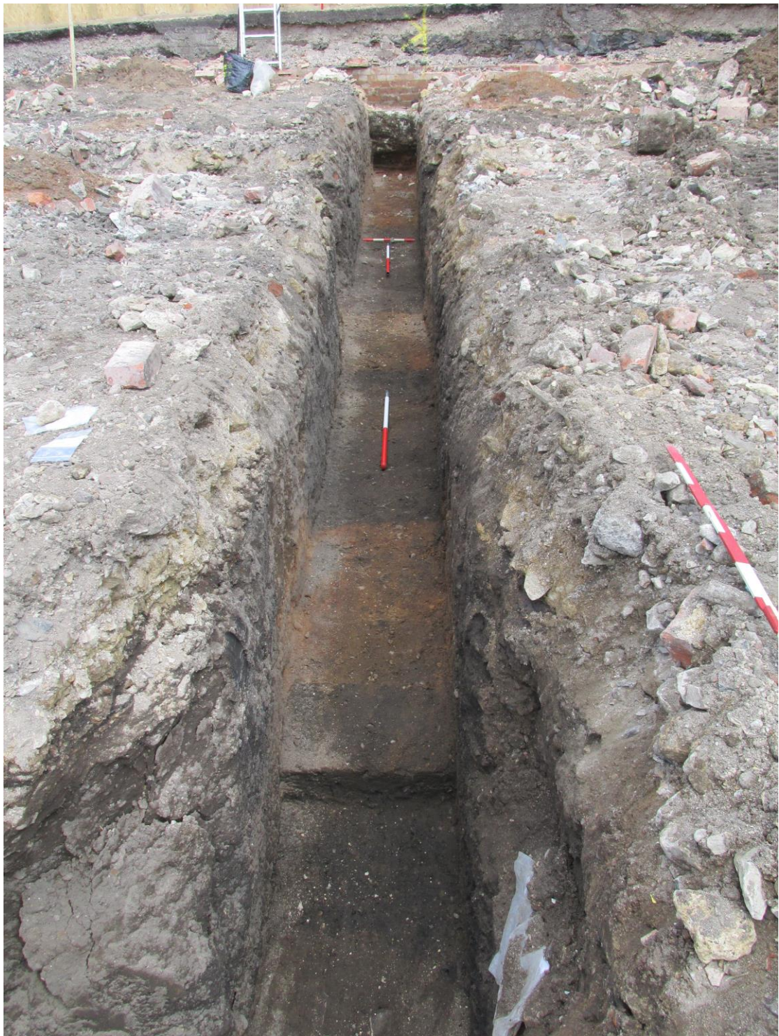
Plate 9; trench 2, from the south showing contexts (pits) 200, 202 & 210. Concrete foundations associated with a brick wall aligned east-west can be seen at the north end of the trench.
