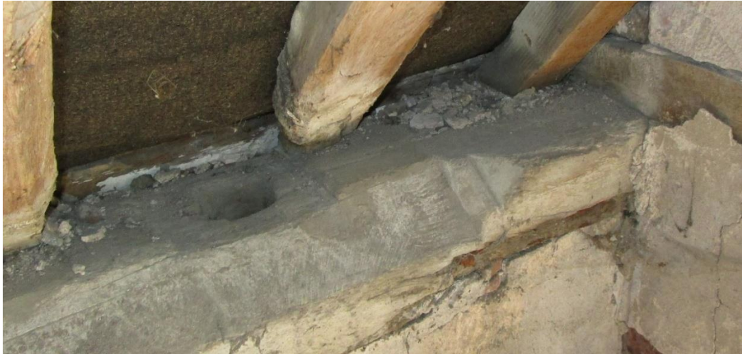
Plate17; Split and re-used beam, with bar-stop, as wall-plate in east-wing of coach-house
