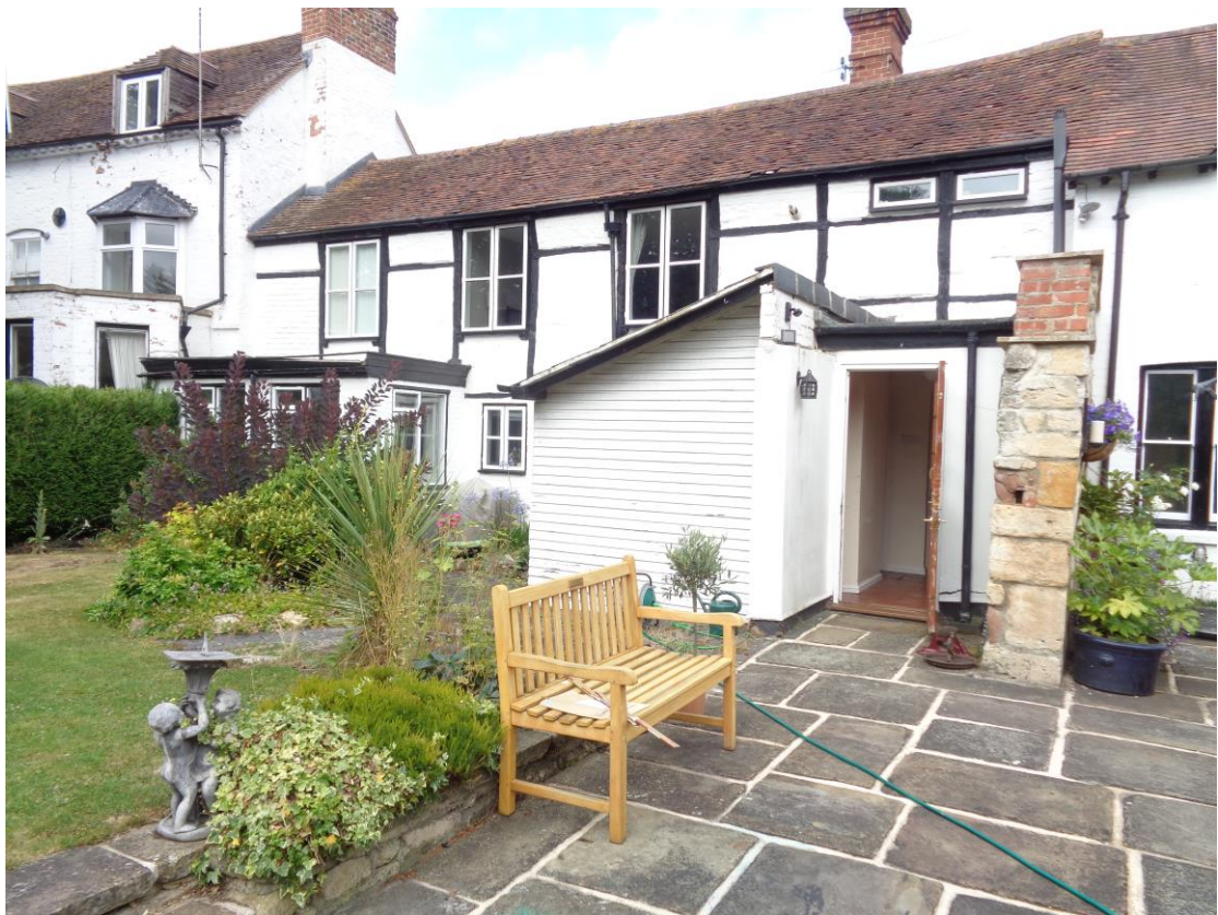
Plate 2; location of the proposed extension. Note the masonry wall on the right
