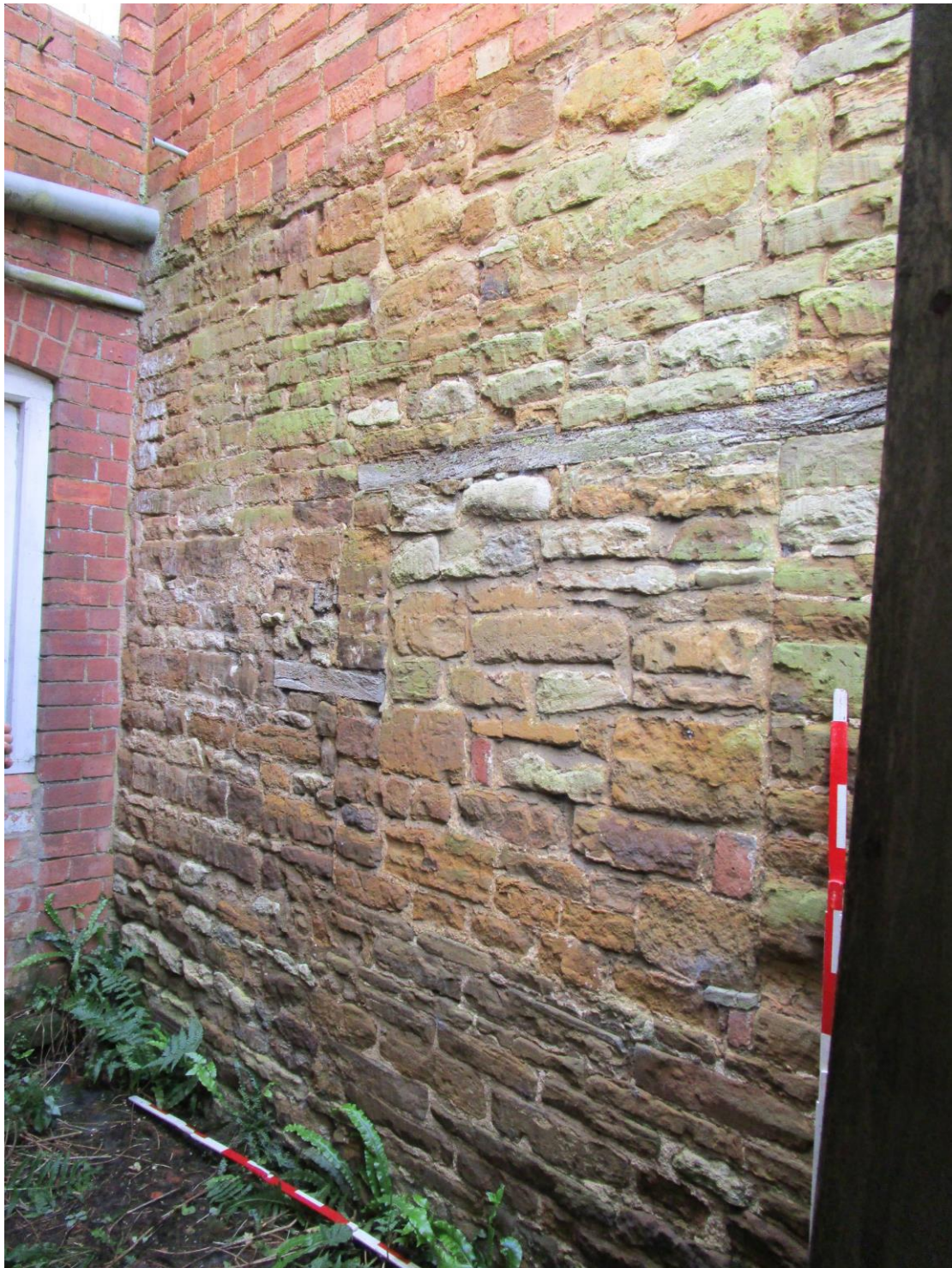
Plate 9; No.28, blocked rear window
