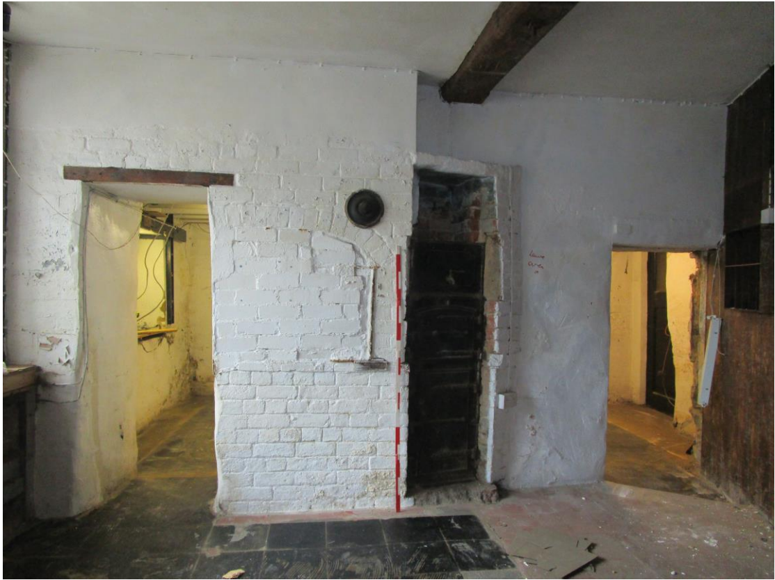
Plate 16; No.28, oven in west bay of original house, cut through by later opening
