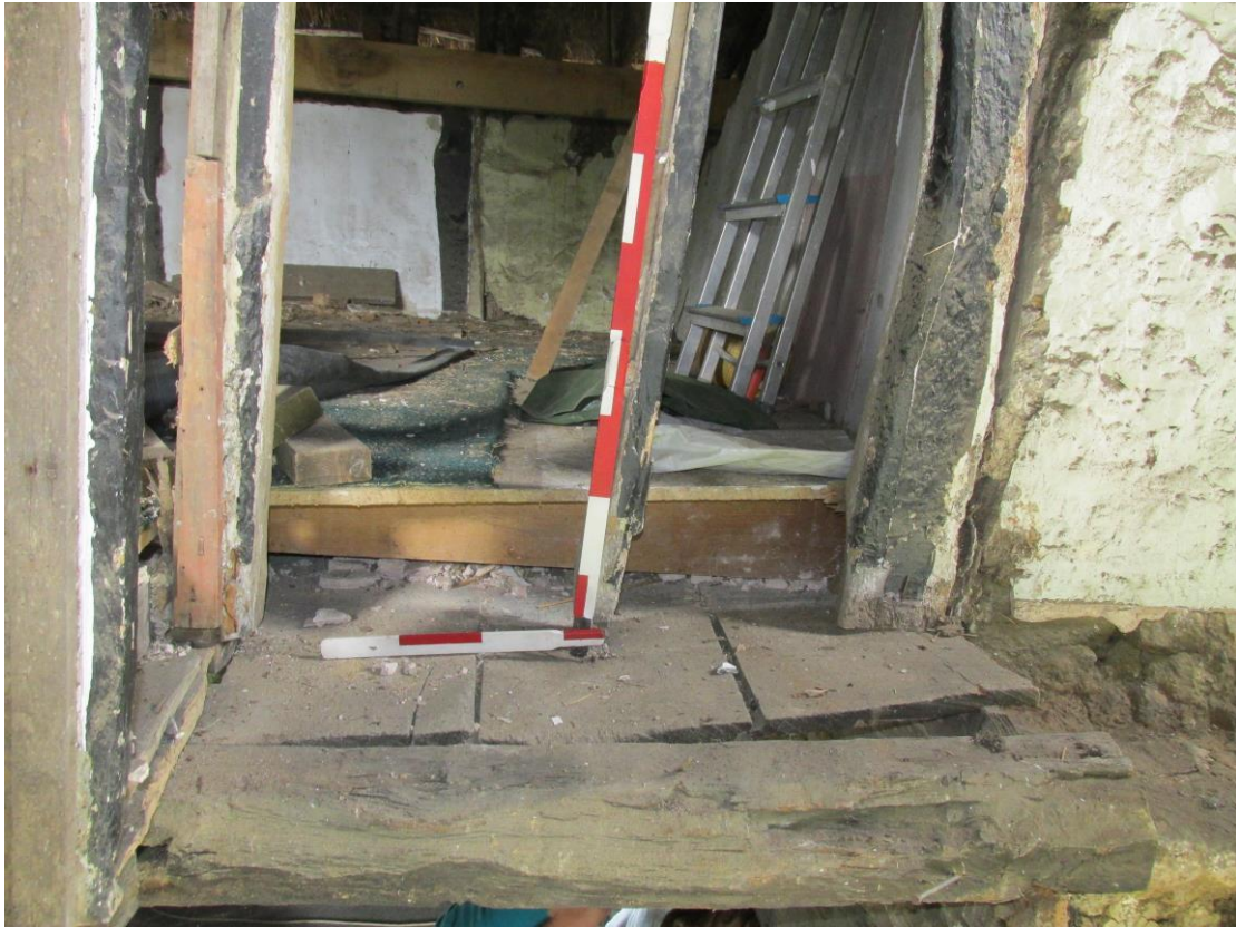
Plate 15; Detail of 1 st floor partition and old floor at corner of chimney from east
