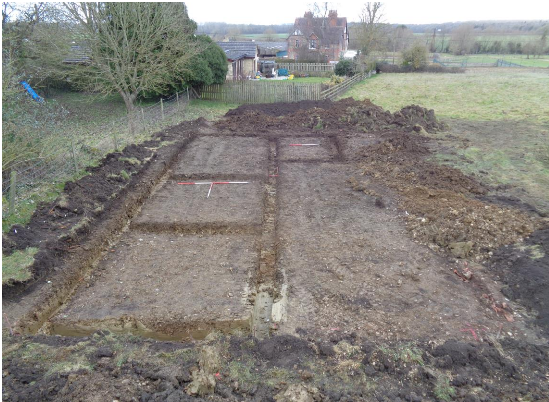
Plate 1; excavation for the proposed stable block (north end of trench 1), view to the north
