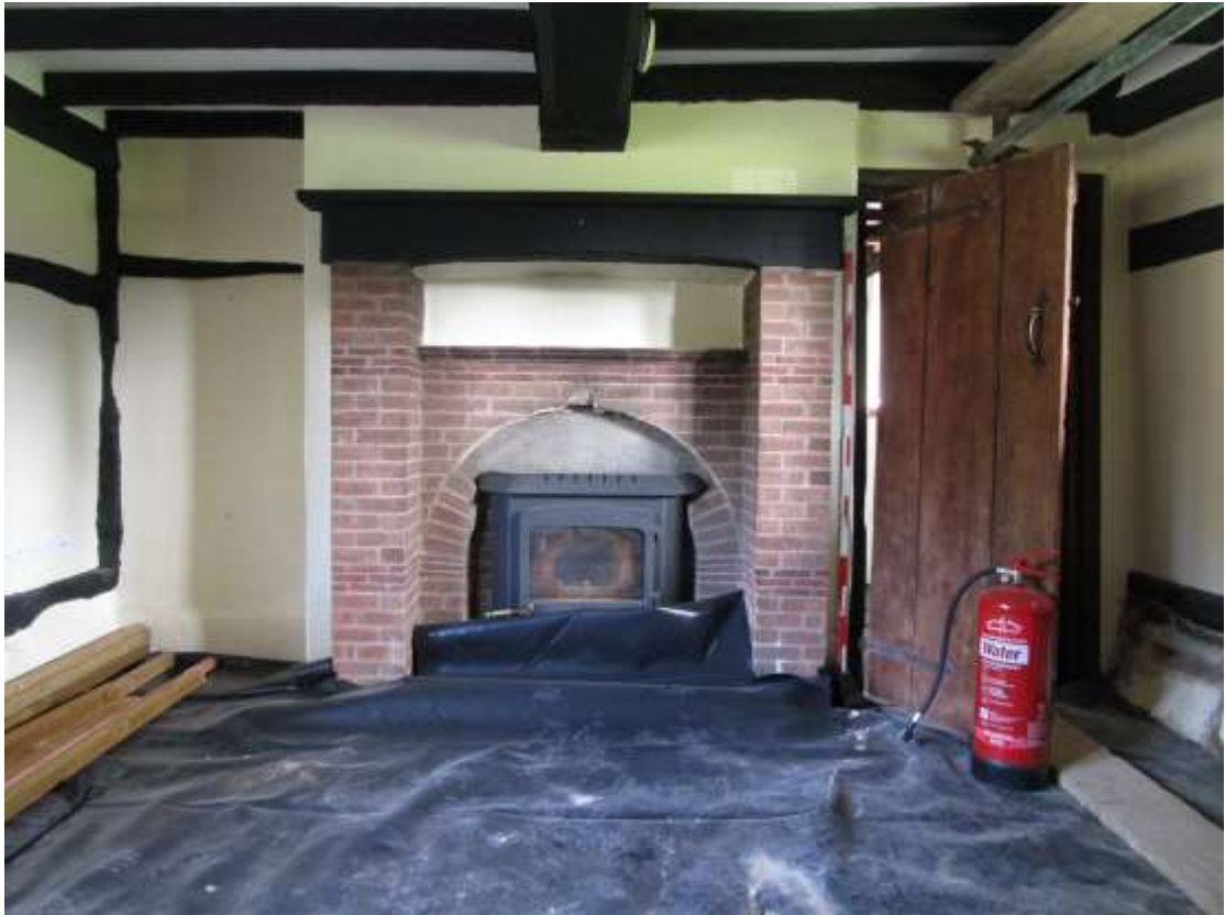
Plate 7; north chimney; early C20 renovation of fireplace, and one of the contemporary C17 style three-leaf doors.
