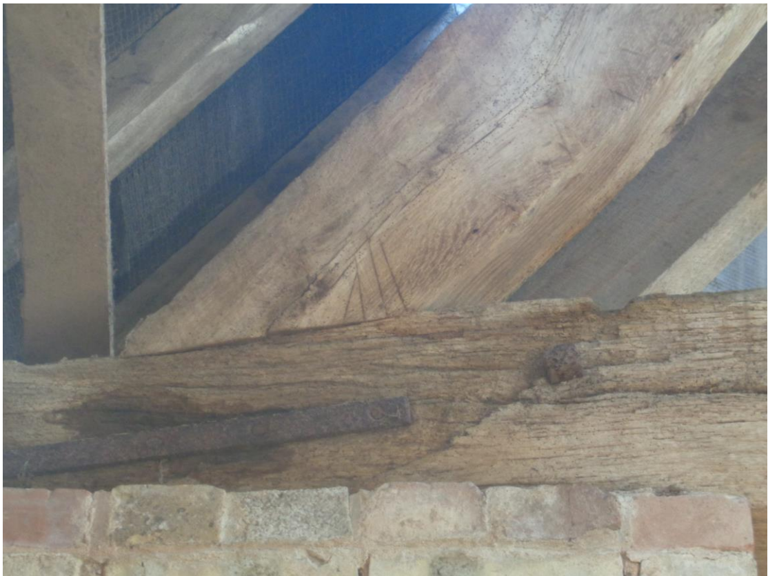
Plate 8; medieval carpenters; marks on the roof truss in the west bay of the threshing barn
