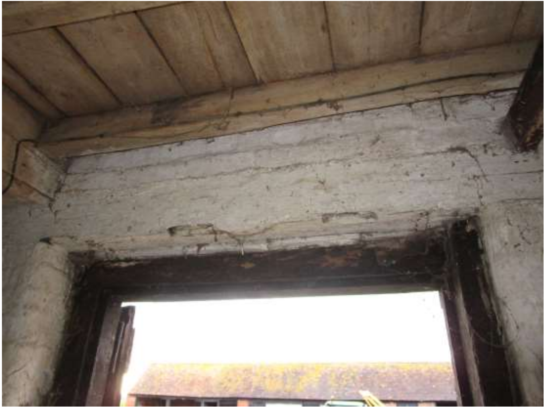
Plate 22; Former stables; Reused wall-plate displaying birds' mouths.
