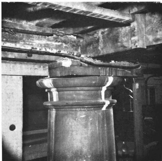
BROKEN LINTEL AND COLUMN CAPITAL SEEN FROM OUTSIDE AND INSIDE THE ENTRANCE TO COUNTY HALL, LEWES
