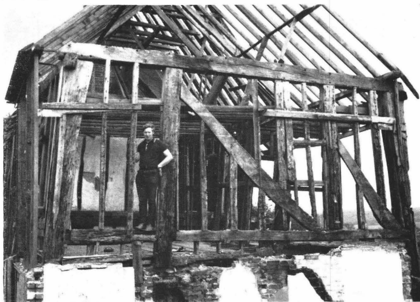
A. Original west wall showing scale of structure and false walling to north elevation
