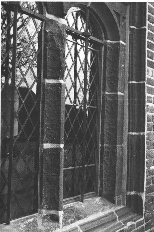
Fig. 33. Laughton Place. Detail of three-light window showing original terracottas and modern replacements.
