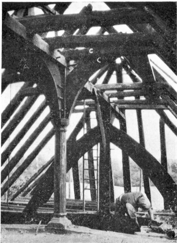
Roof, looking E. (The wall between the hall and the room over the screen passage is removed: braces show its position.)
