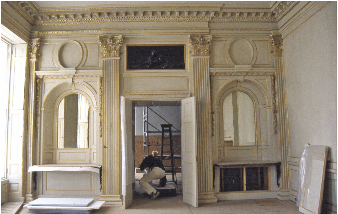
Fig. 29. The joinery at the south end of the Dining Room, during restoration.
