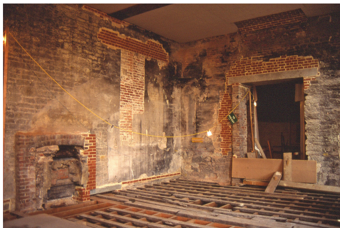
Fig. 23. The Dining Room, looking northwest after the fire and following the removal of the surviving panelling and floorboards. Note the blocked window opening to the right of the fireplace.
