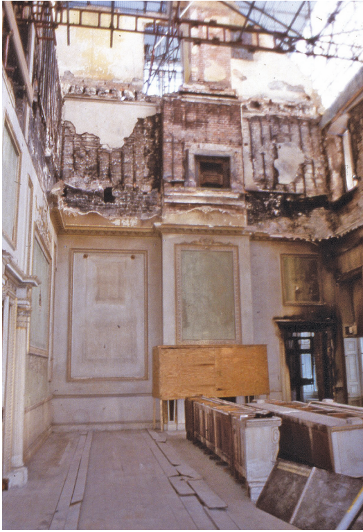
Fig. 46. The Saloon after the fire, looking east.
