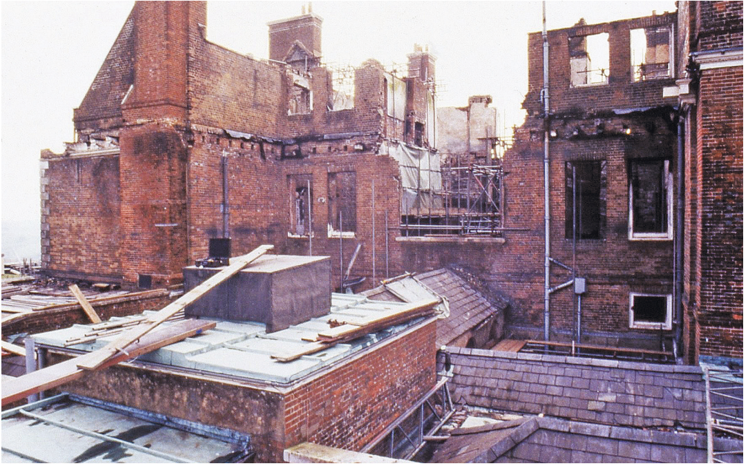
Fig. 19. The north side of the house, after the fire in August 1989.
