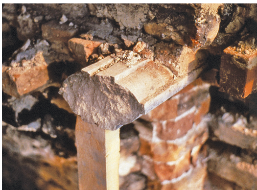
Fig. 8. A reused stone window mullion from another building, incorporated in the original masonry.
