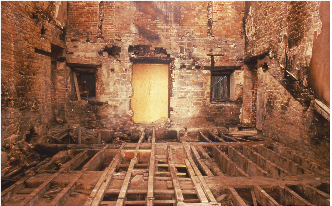
Fig. 20. The north wall of the stairs hall at ground- and first-floor levels, after the fire and the removal of what survived of the staircase, the floorboards and some other joinery.
