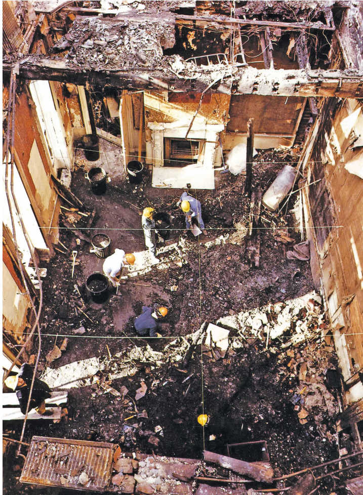
Fig. 2. Salvage excavations in the Red Drawing Room, after the fire. Note the string grid at ceiling level which enabled finds to be located within the space.
