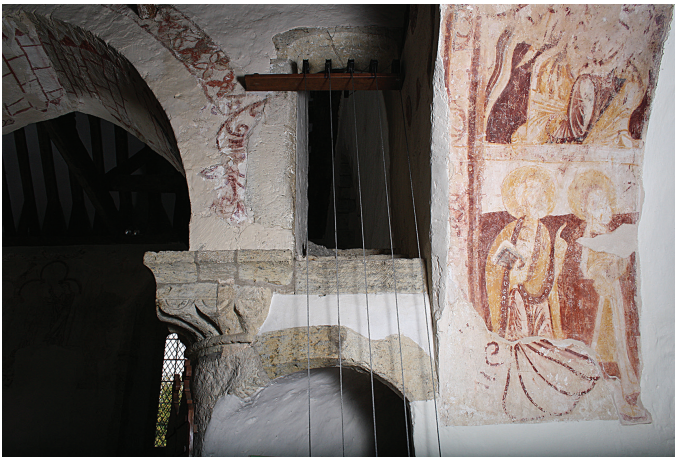
Fig. 14. E. end of nave arcade viewed from aisle, with patterning [B]; entrance to rood loft and squint; holy figures in soffit of aisle arch [A]; below, indeterminate lines [?E].
