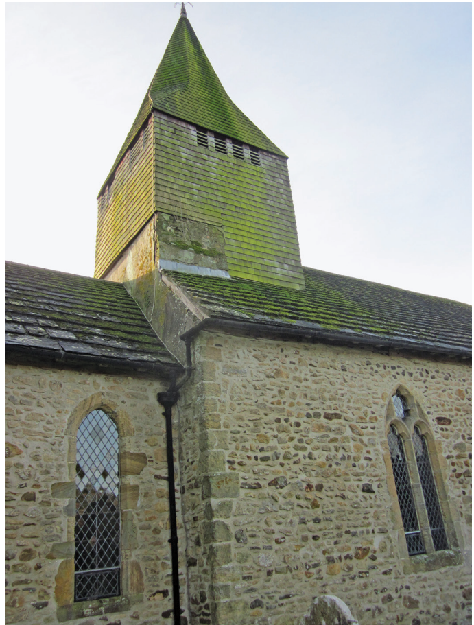
Fig. 3. View of West Chiltington church from the north-east: the central tower and spire are visible. The masonry on the east side once supported an earlier bell-turret. The north-east nave quoin created in Pulborough Stone is also visible and the slightly more pronounced, centrally placed, stones are set in Anglo-Saxon style.
