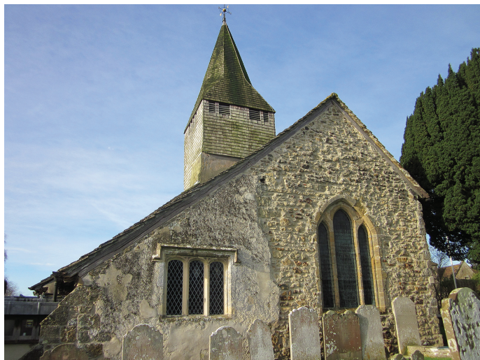
Fig. 6. The east face of the church is partially covered with render, largely removed to the north of the south-east chancel quoin (of which a few stones only are visible).
