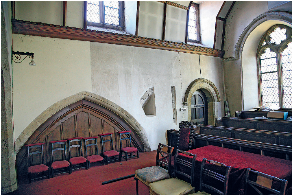
Fig. 2: Petworth, St Mary: remains of reveal of single-light window in west wall of north transept at gallery level (photo: D. Parsons).
