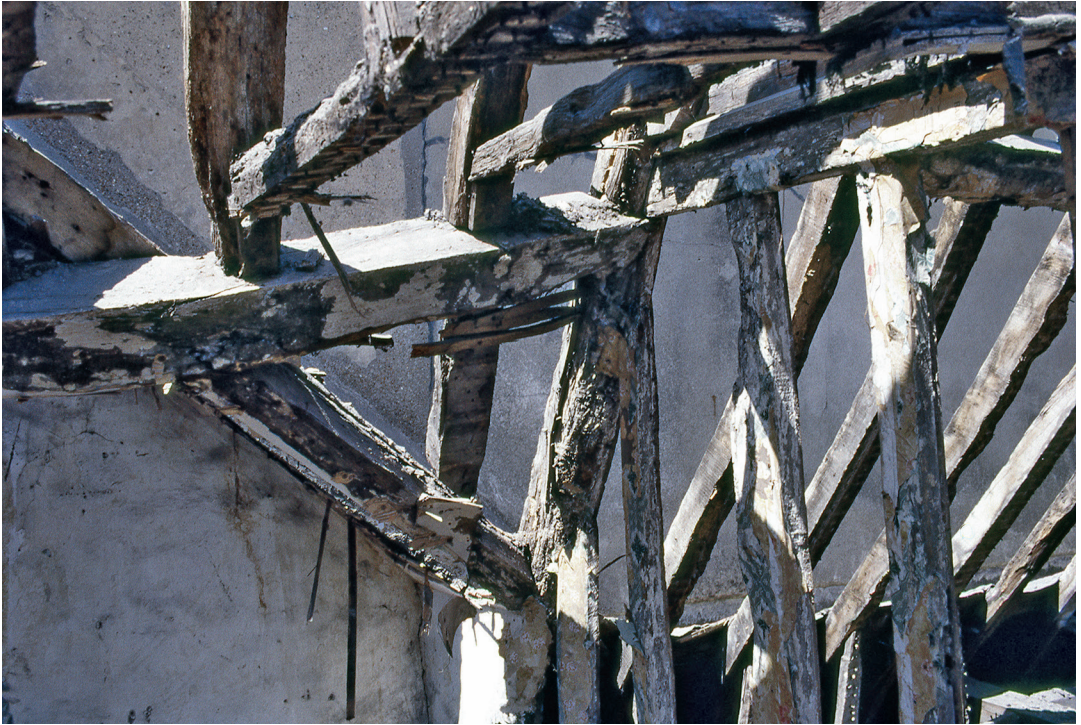
Fig. 27. North end of west butt purlin at roof truss F1-F2, with in situ valley rafter and jointed-in jack rafter filling the gap between valley and purlin.
