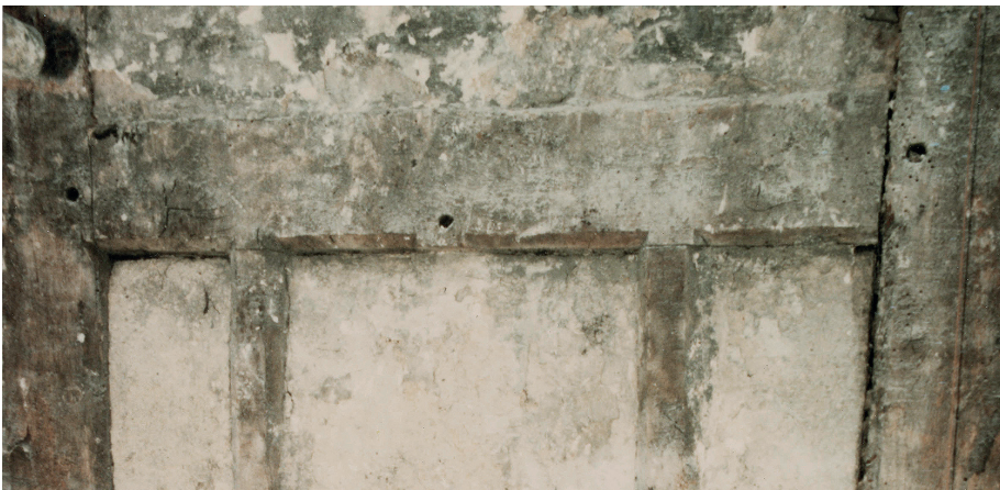
Fig. 12. Truss A-A, blocked hall window: detail showing stopped chamfers on window head and jambs, plus two surviving chamfered mullions.
