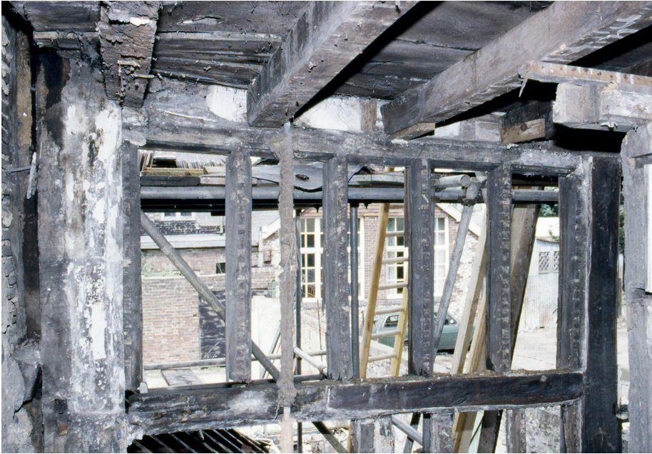
Fig. 17. West five panes of the frieze window which extended across the full width of the Phase 2b north elevation. The window's cill doubles as the wall's midrail, whilst the joists supporting the garret floor are supported on the window's head.
