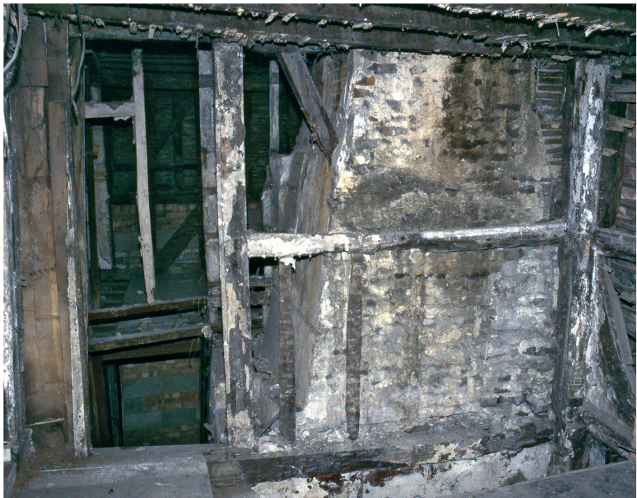
Fig. 18. West wall of Phase 2b range: note doorway at south (left) end.
