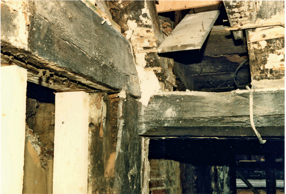
Fig. 15. Tie-beam B-B, head of principal post B1, and wall-plate to bay A-B, the latter supporting a few surviving Phase 1 rafter fragments. That on the left is part of the surviving rafter pair and is halved over the east face of the tie-beam.
