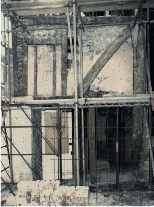
Fig. 11. Truss A-A: east elevation showing foot-brace (upper right), and blocked hall window (upper left).
