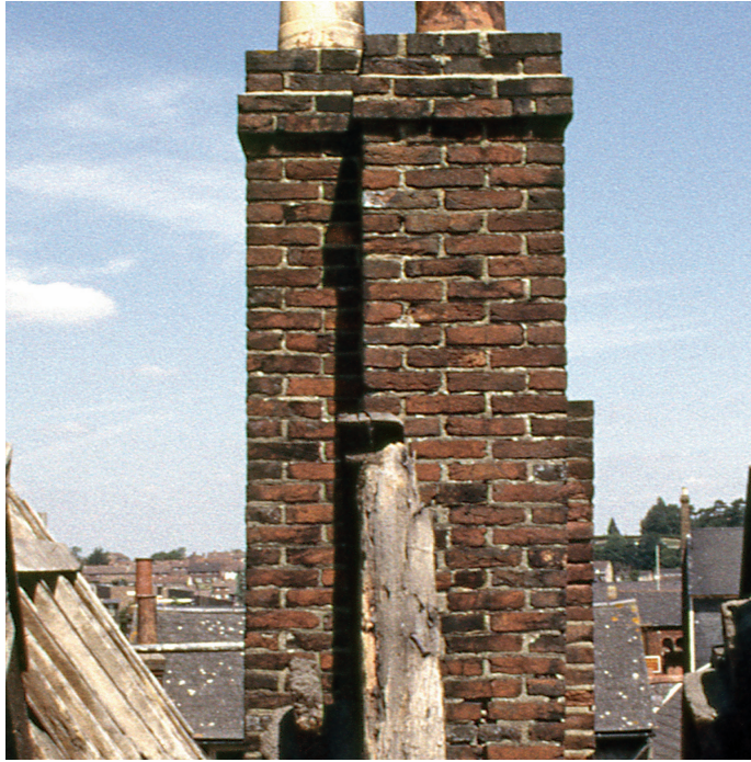
Fig. 19. Phase 3 chimney cap from south showing likely Phase 2b flue projecting from east (right) face.
