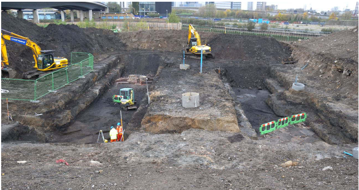
Trench 2 (left), looking west, with timber baseplates with concrete [32] & [33] and timber sleepers (front) and brick structure [31] (rear)
