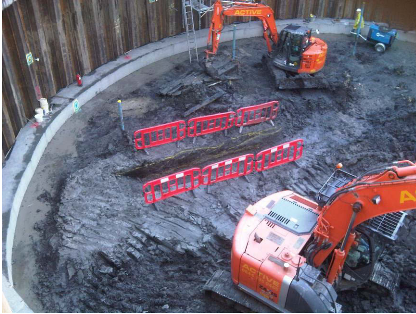
Photo 7 Auxiliary Shaft, showing trench excavated for investigation of the alluvial silt and gravel interface and section recording - looking south-west
