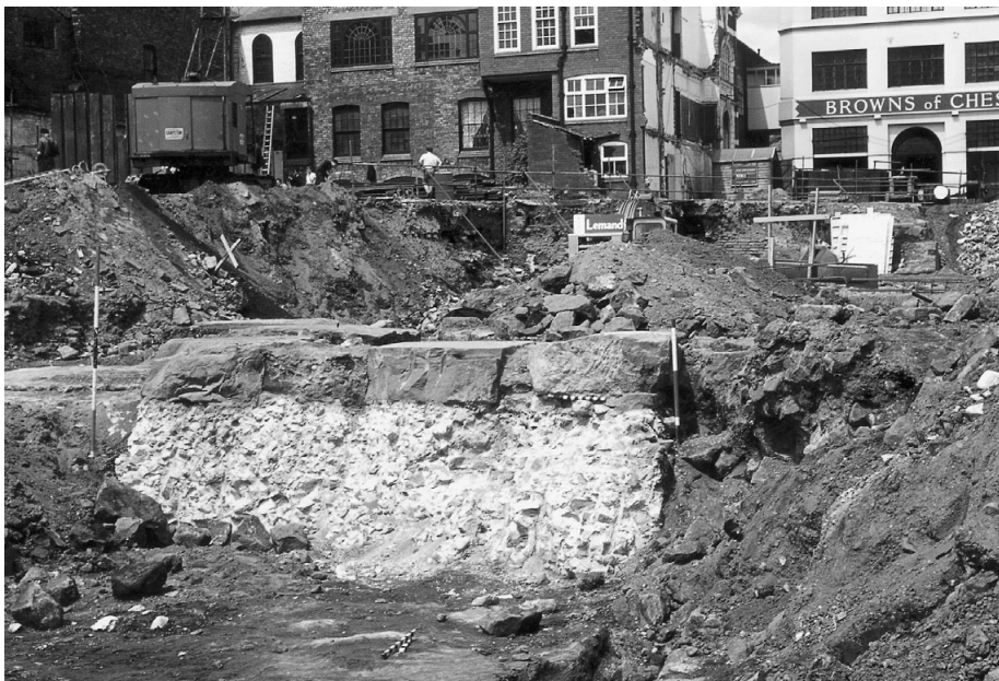
III VIII.9 Concrete bases which supported the main reservoir for the fortress baths, photographed during destruction in 1963 to make way for the Grosvenor Shopping Centre. (Copyright Chester City Council)
