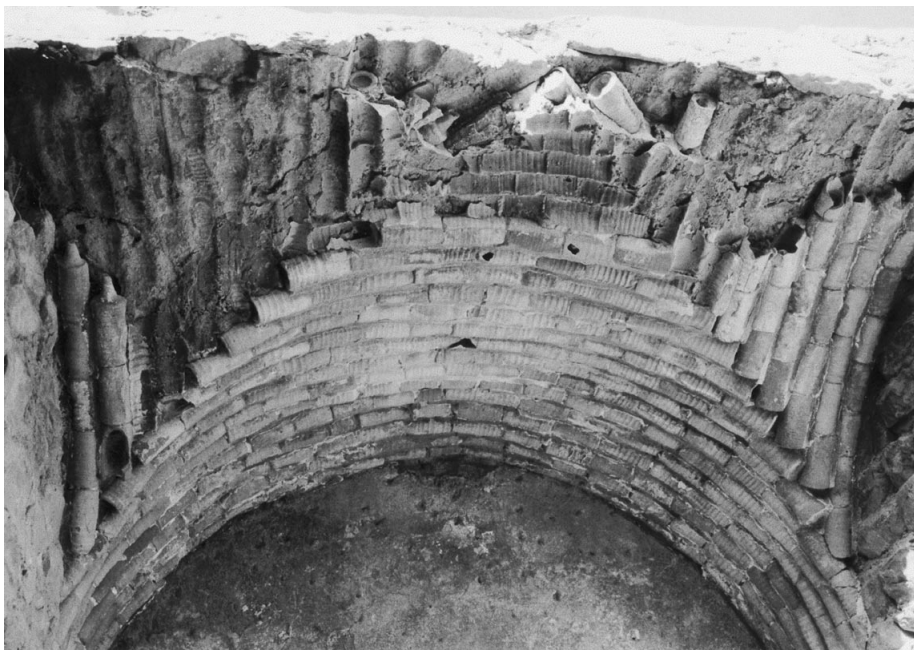
III VIII.12 Examples of tubi fittili in position used as inner lining of vault at Bulla Regia, Tunisia. (Photo courtesy T J Strickland)
