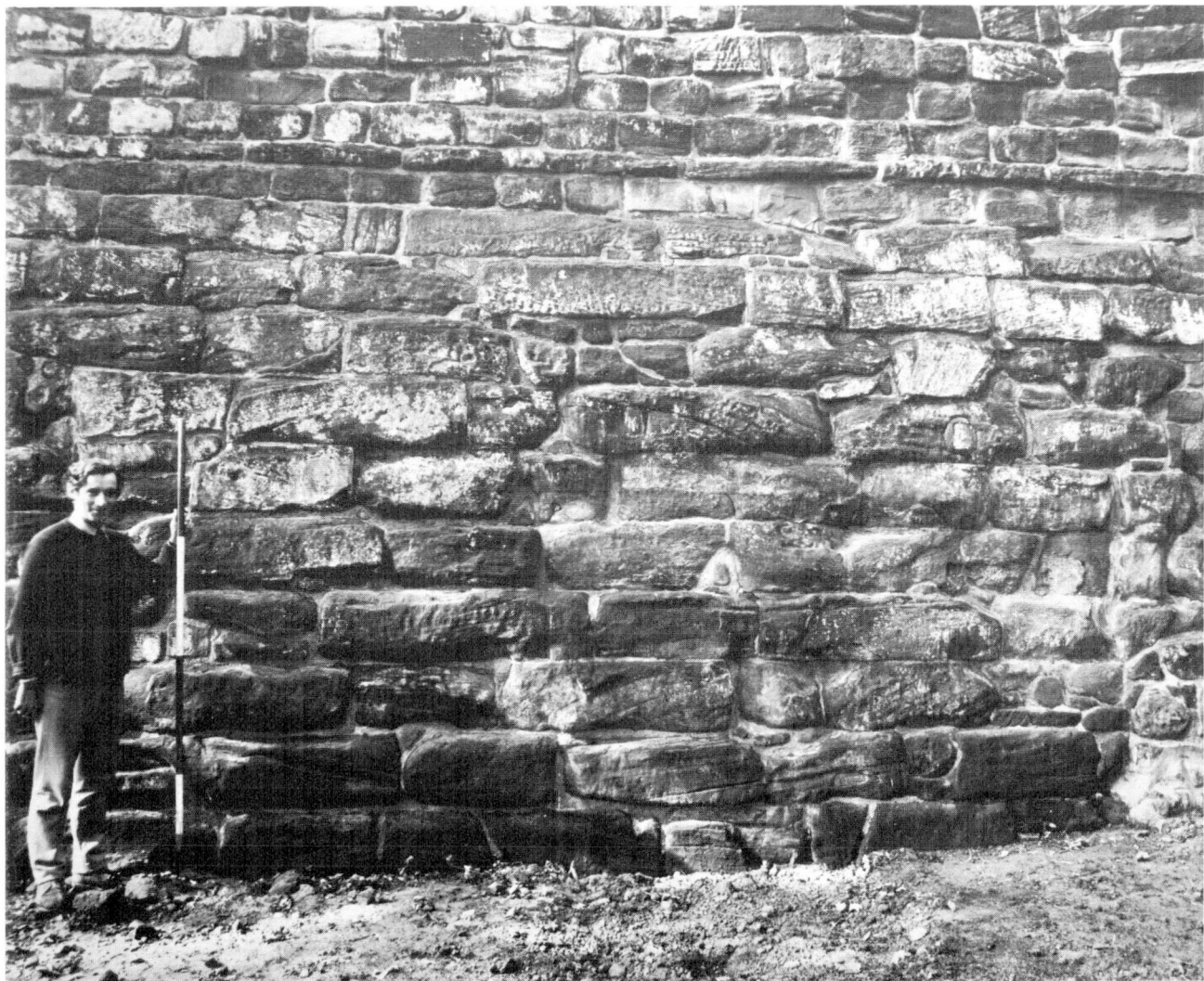
Plate 1 — The East face of the City Wall approximately fifty metres North of the Kaleyad Gate. Although worn, damaged and subsequently repaired in modern times, the characteristic Roman masonry is clearly visible. (Two metre scale).
