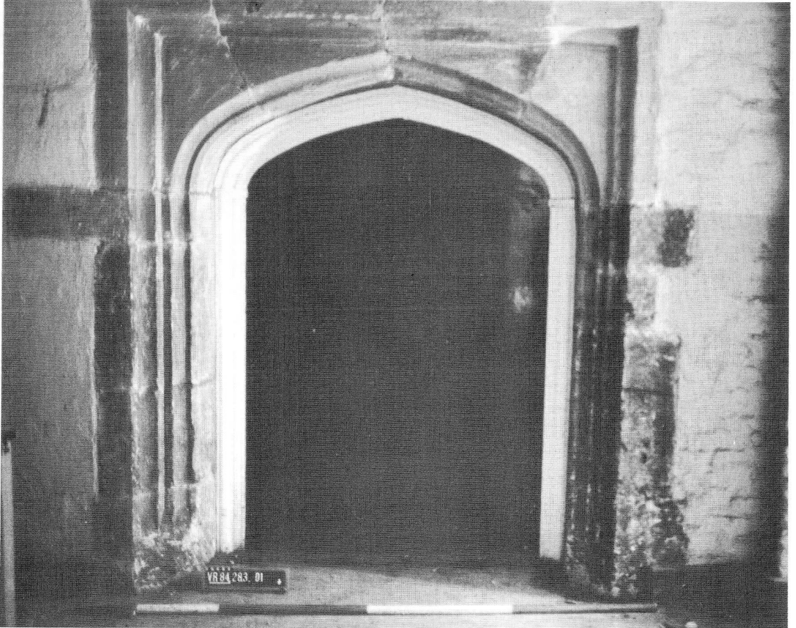
Fig. 7: The doorway to the kitchen from the line of the cloister walk.
