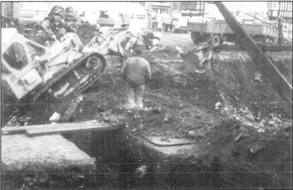
17 Contractor's excavation of the basement car park on the Old Market Hall site after the end of archaeological work.
