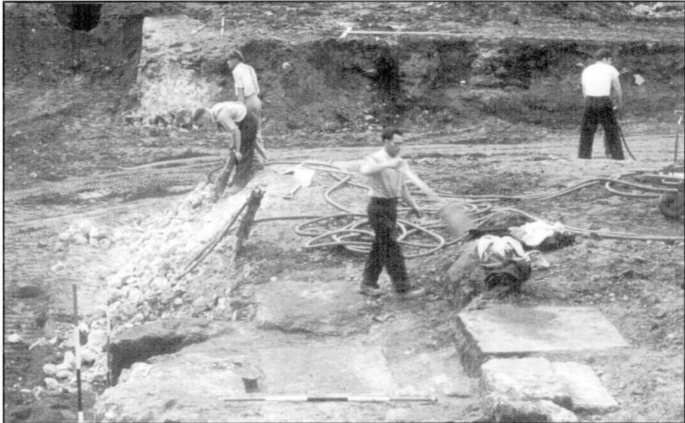
14 The south-east corner of the Roman legionary bath building, as exposed and destroyed in 1964. The concrete base in the centre being demolished with a pneumatic drill was the foundation for the water tank.
