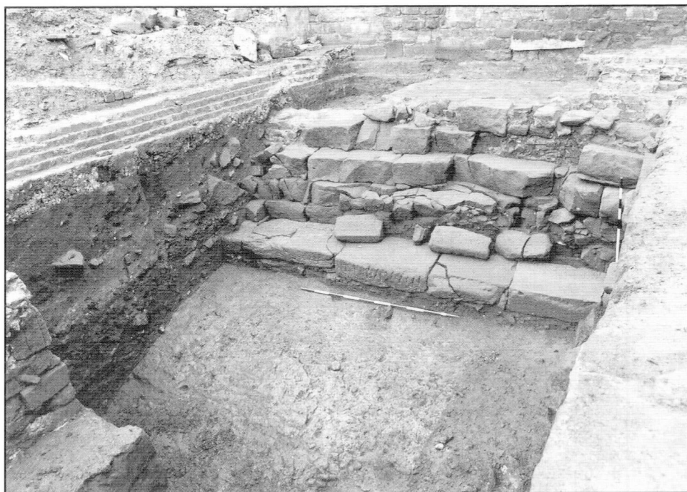
II.4 St John Street 1988/9: fracturing of the Roman wall face caused by forward collapse
