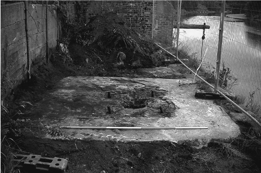
III. V.1: Concrete crane base with central pivot-hole, surrounded by in-situ fixing bolts. Looking southwest. Two metre scale
