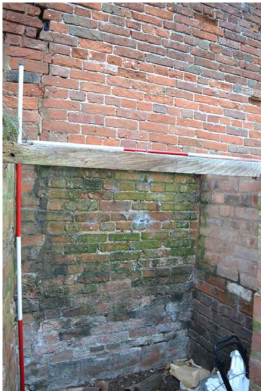
Plate 11: West elevation, anomalies in the brickwork
