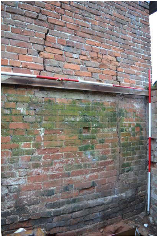
Plate 10: West elevation, anomalies in the brickwork
