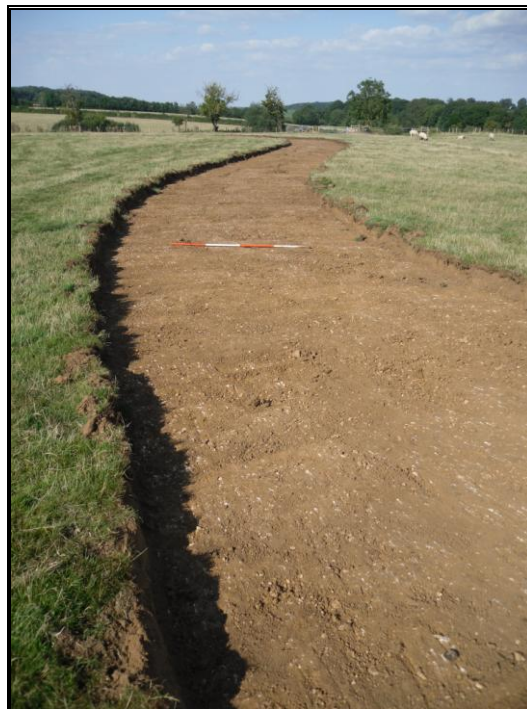
Figure 5. The roadway area with topsoil removed on the eastern part of the site
