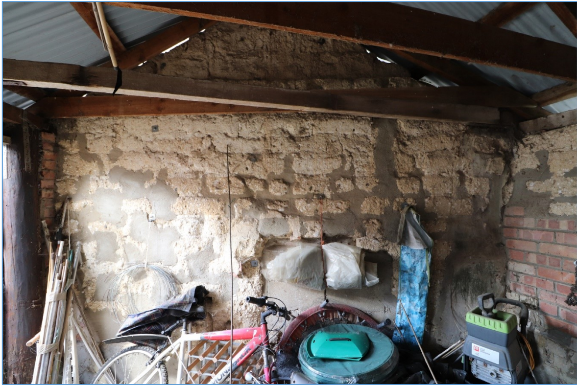
Figure 44. The interior of the northern gable of the northern extension, looking north.
