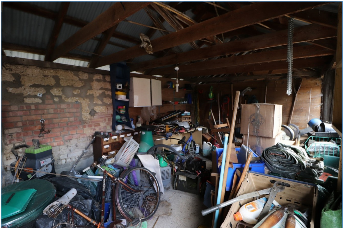
Figure 43. The interior of the northern cell of the northern extension, looking south-east.
