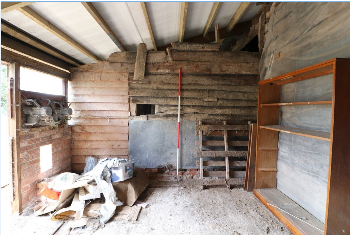
Figure 35. The western elevation of the eastern bay of the southern lean-to, looking west, showing surviving weatherboarding contemporary with the covering of the barn and the rebuilt southern wall.
