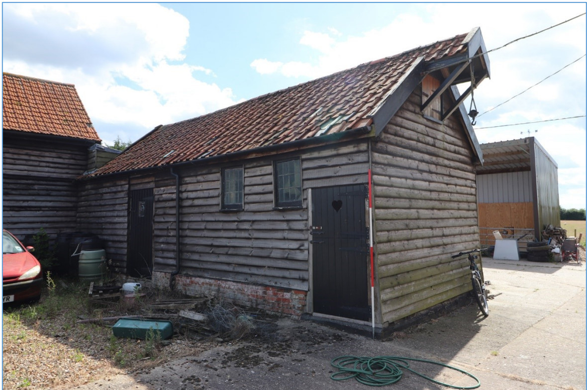
Figure 52. The exterior of the small barn, looking south-west, showing the modern weatherboarding and the gable pulley mechanism.
