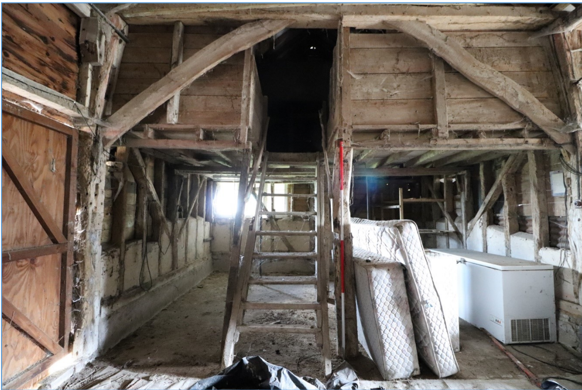
Figure 21. The eastern elevation of the central bay, looking east, showing the stairs leading up to the upper storey.
