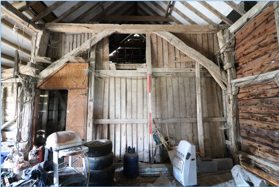
Figure 16. The western elevation of the central bay, looking west, showing the timber partition between the central and western bays.
