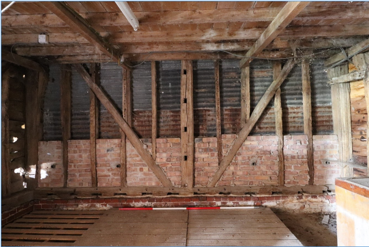
Figure 20. The western elevation of the western bay, looking west, showing the surviving timber framing, brickwork and corrugated metal sheeting.
