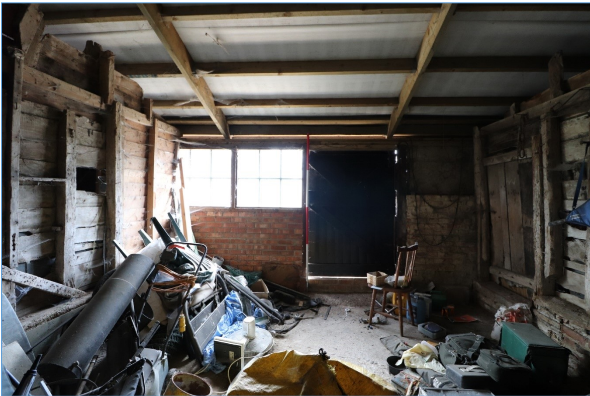
Figure 28. The southern elevation of the central bay of the southern lean-to, looking south, showing the later bricking up, openings and the new roof.
