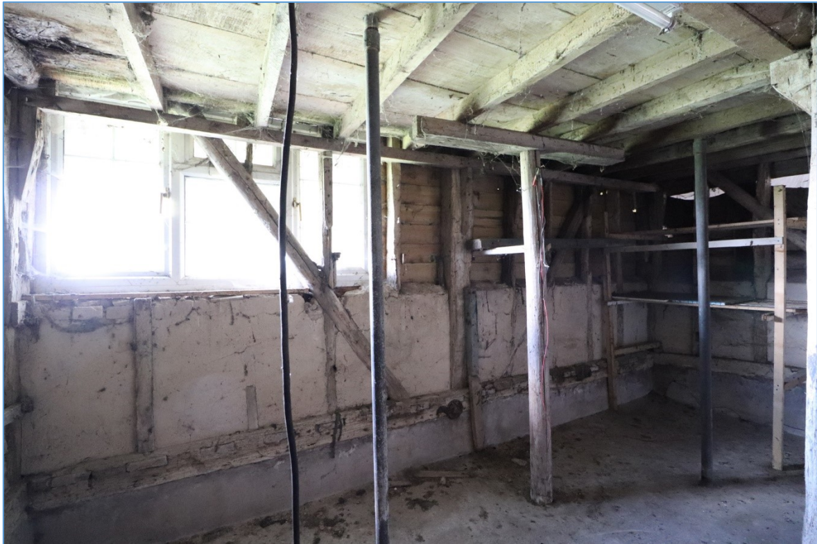
Figure 26. The eastern elevation of the eastern bay, looking east, showing the surviving timber framing with render infill and modern window.
