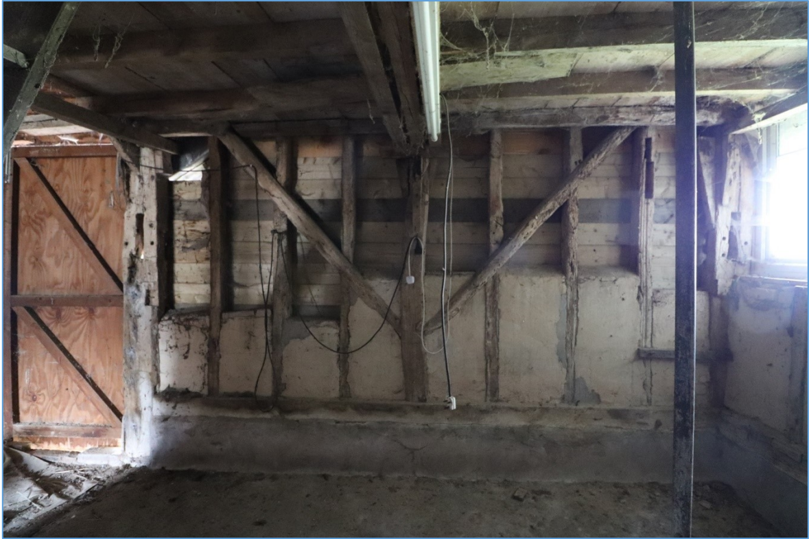
Figure 24.. The northern elevation of the eastern bay, looking north, showing the surviving timber framing with render infill.
