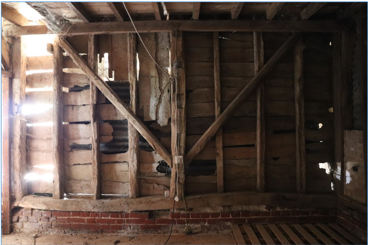
Figure 19. The southern elevation of the western bay, looking south, showing the surviving timber framing.
