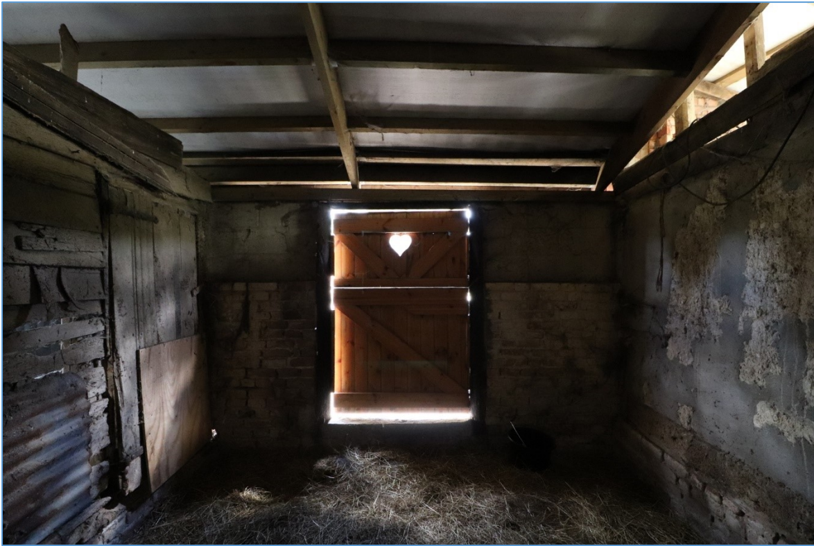
Figure 33. The southern elevation of the western bay of the southern lean-to, looking south, showing the mixed building phases and inserted stable door. .
