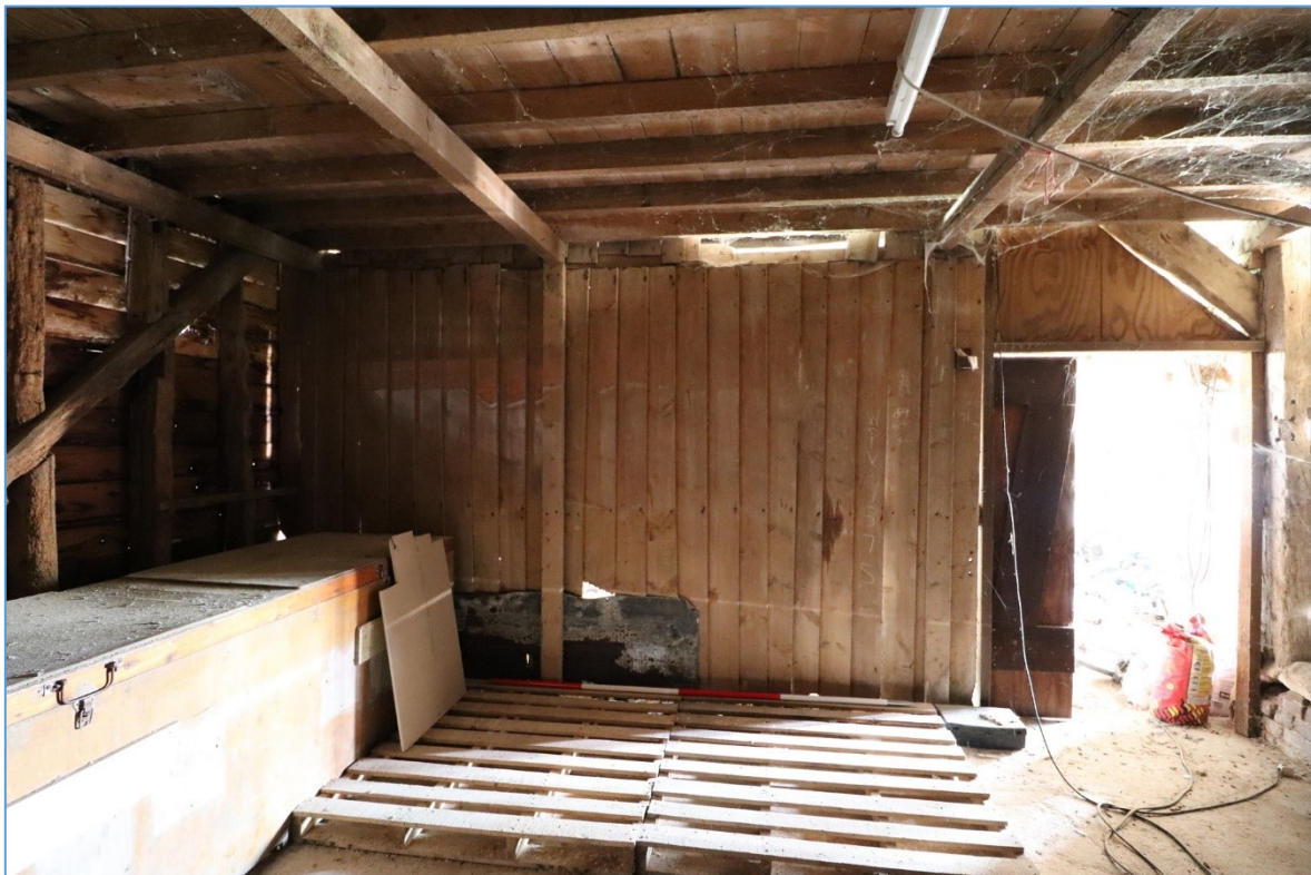
Figure 17. The eastern elevation of the western bay, looking east, showing the timber partition and inserted upper floor.
