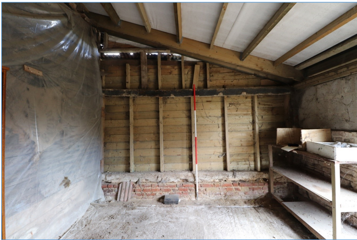
Figure 37. The eastern elevation of the eastern bay of the southern lean-to, looking east, showing the rebuilt timber walling atop an older sill beam and plinth.
