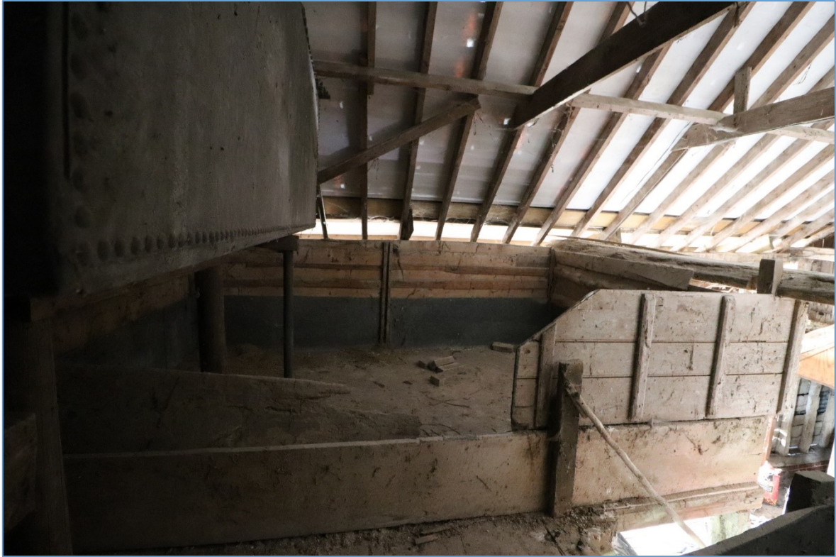
Figure 22. The upper storey of the eastern bay, looking south, showing timber hopper and lead water tank.
