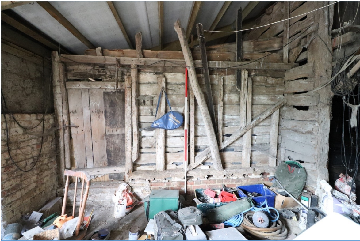
Figure 29. The western elevation of the central bay of the southern lean-to, looking west, showing surviving timber-framing from the original porch of the main barn.
