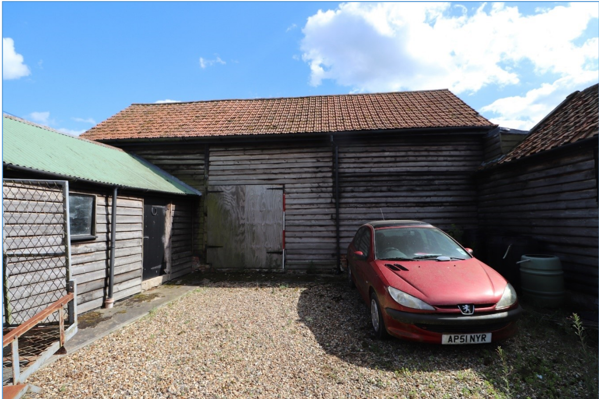
Figure 14. The exterior of the northern elevation of the main barn, showing the blocked former central doorway and modern weatherboarding of the exterior.
