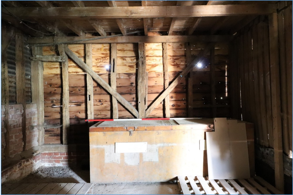
Figure 18. The northern elevation of the western bay, looking north, showing the surviving timber framing with modern weatherboarding attached.
