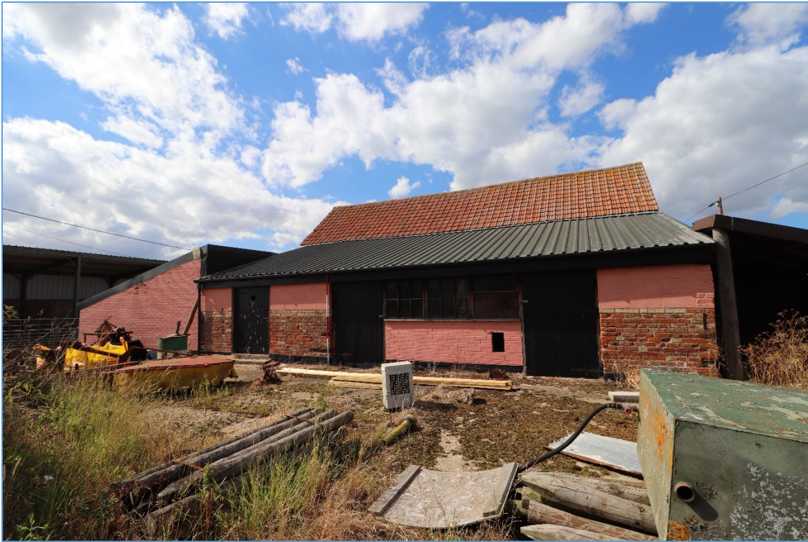
Figure 27. The southern wall of the southern lean-to, looking north, showing the various openings and different construction methods in evidence.
