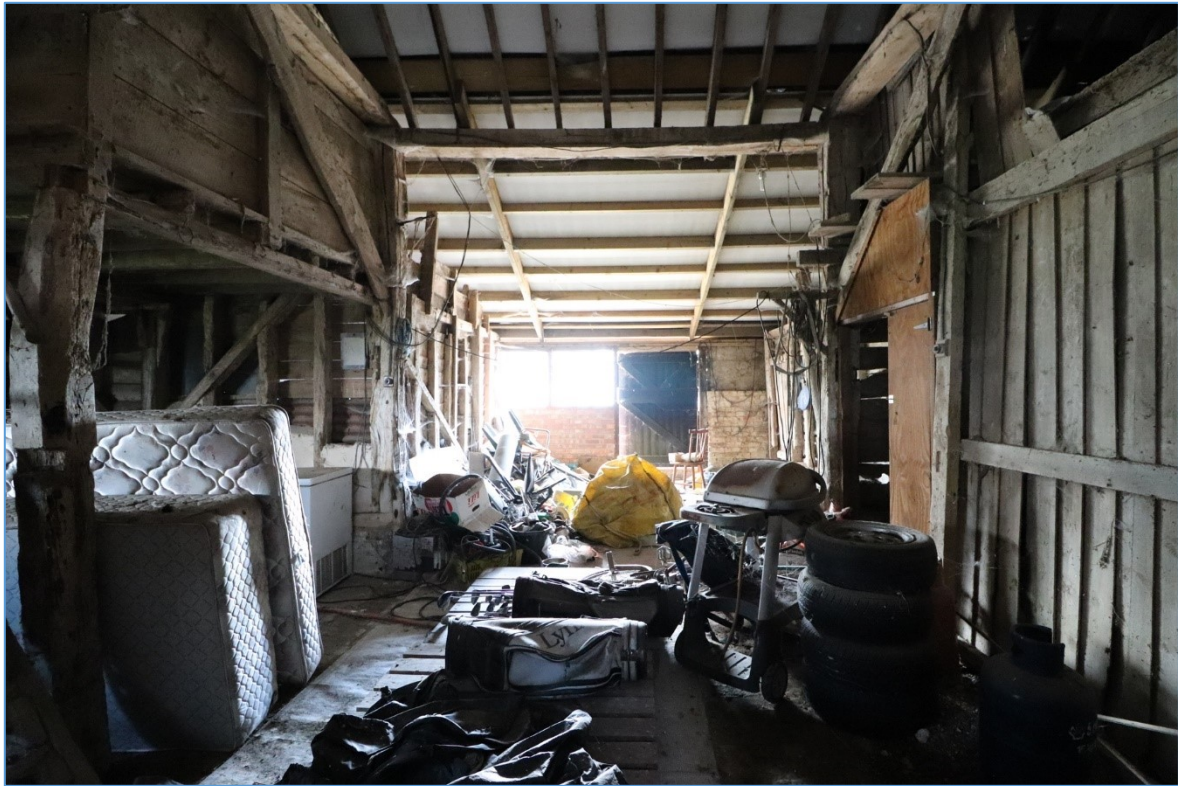
Figure 15. The central bay of the main barn, looking south, showing the connection with the southern lean-to.
