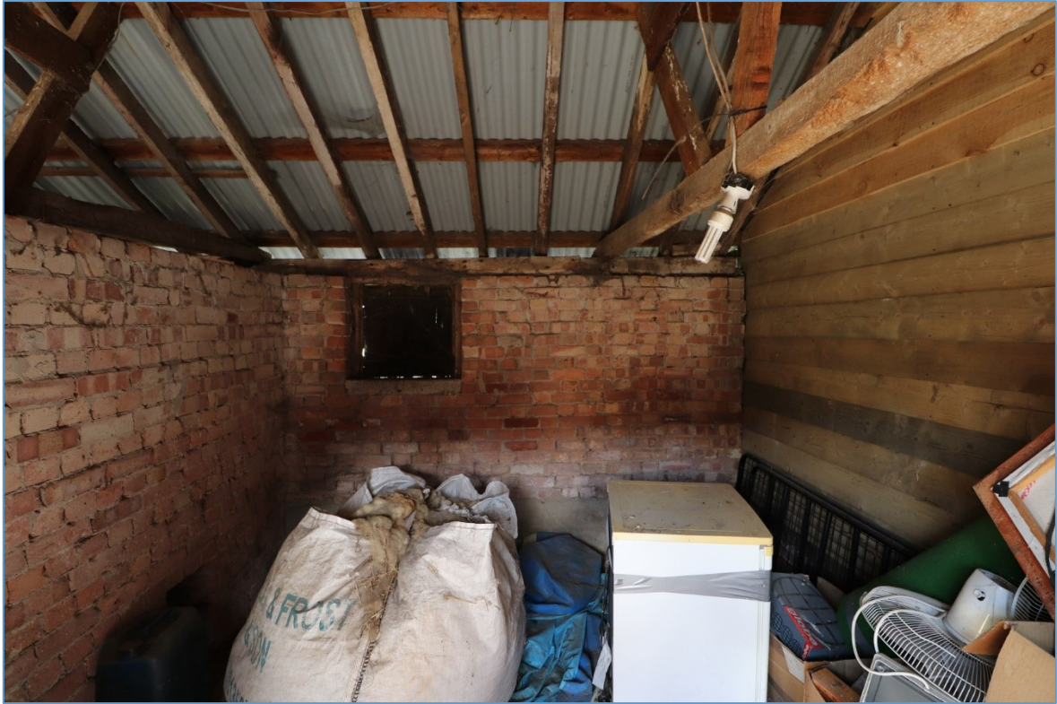
Figure 42. The interior of the southern cell of the northern extension, looking east.
