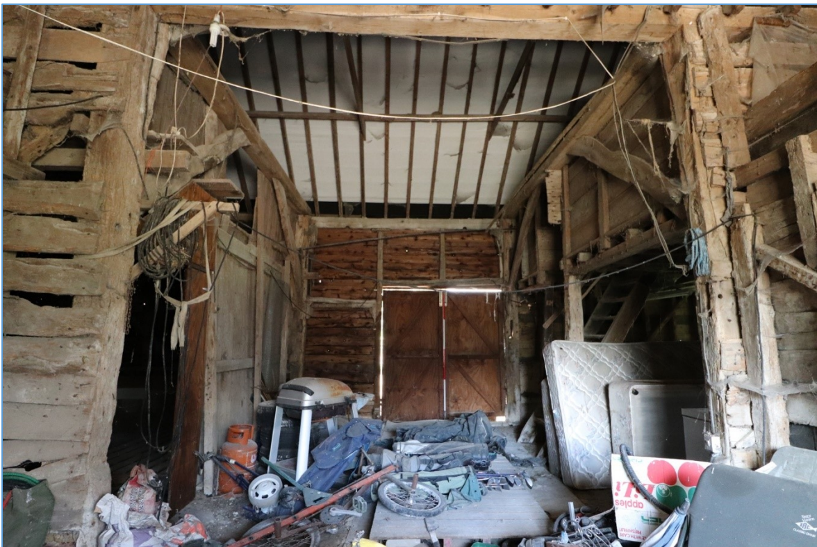
Figure 13. The central bay of the main barn, looking north, showing the position of the former double-doors and cross-frames.
