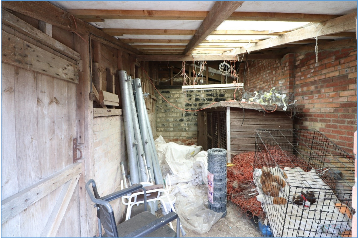
Figure 47. The interior of the southernmost cell of the south-western infill, looking east.
