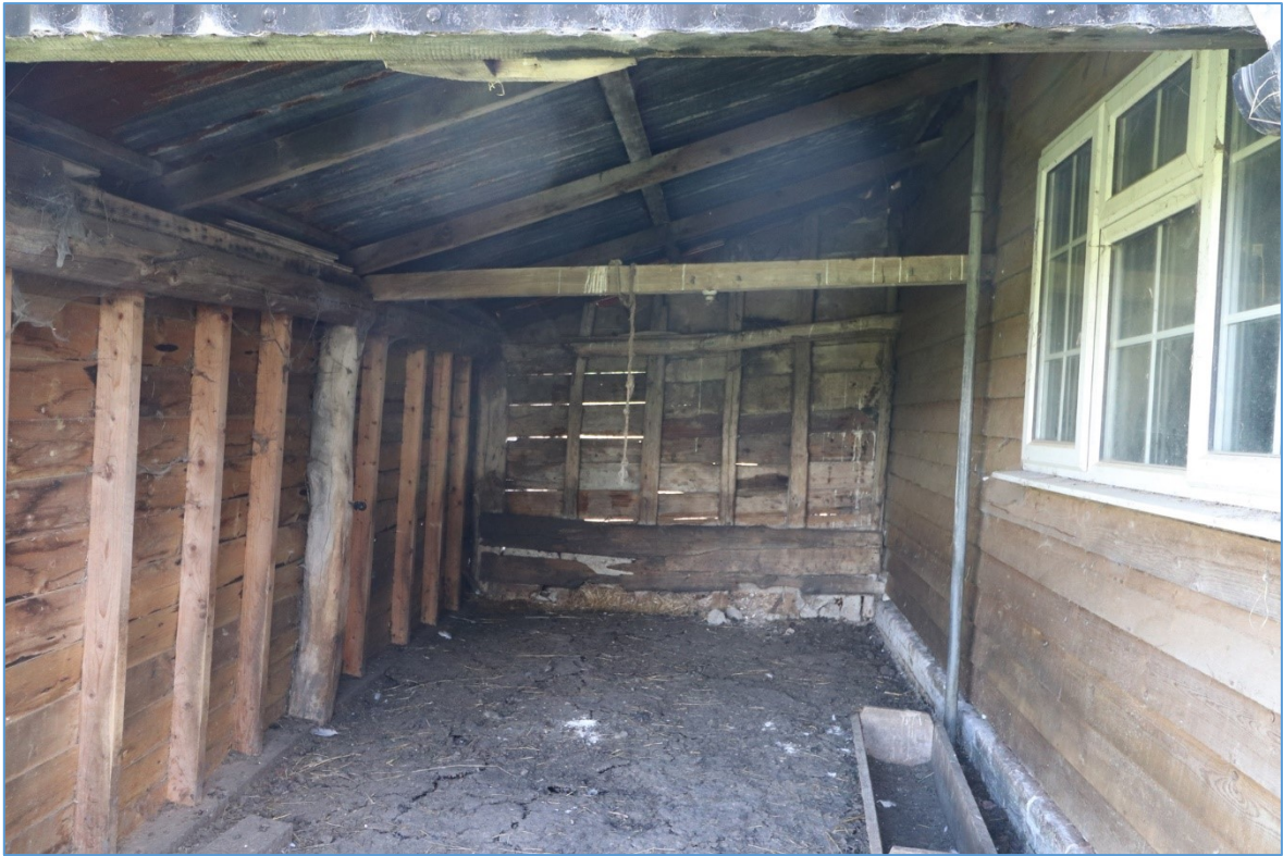
Figure 38. The interior of the northern half of the eastern lean-to, looking south.
