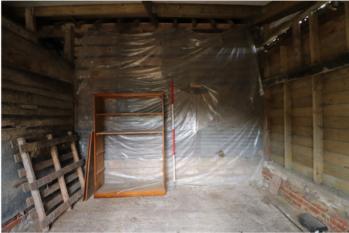
Figure 36. The northern elevation of the eastern bay of the southern lean-to, looking north, showing the surviving weatherboarding of the barn behind protective coverings.
