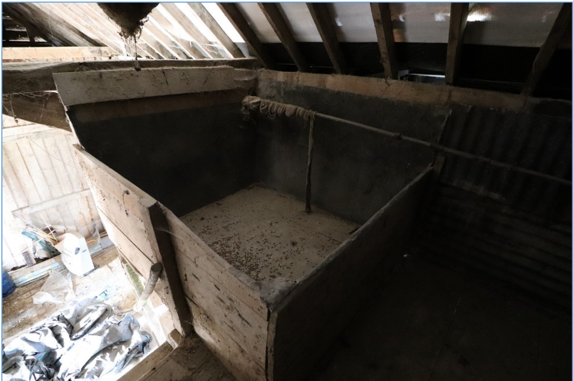
Figure 23. The upper storey of the eastern bay, looking north, showing timber hopper and disused water pipes.
