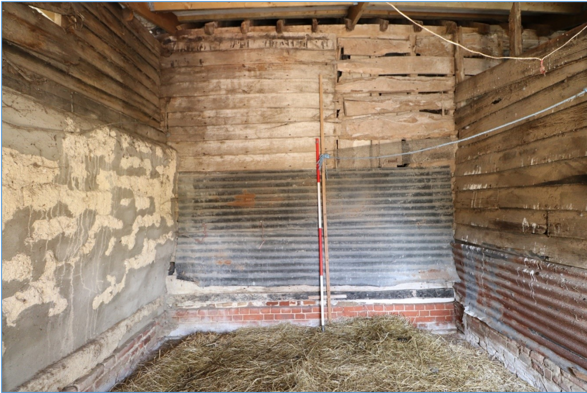
Figure 31. The northern elevation of the western bay of the southern lean-to, looking north, showing the surviving weatherboarding of the barn.
