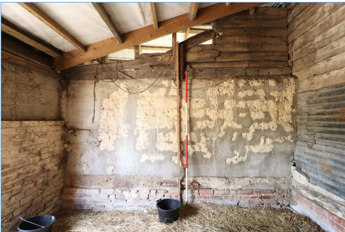
Figure 32. The western elevation of the western bay of the southern lean-to, looking west, showing surviving the rendered timber-framing and weatherboarding above. .
