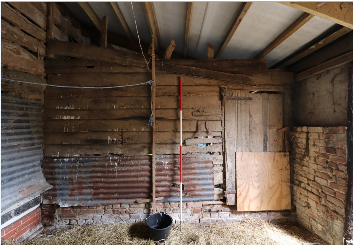
Figure 30. The eastern elevation of the western bay of the southern lean-to, looking east, showing surviving weatherboarding contemporary with the covering of the barn.
