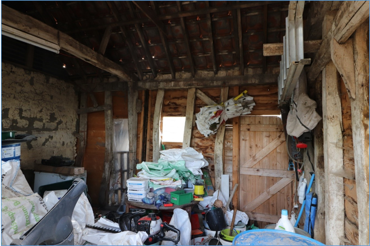
Figure 53. The western wall of the northern half of the smaller barn, looking west, showing the surviving timber framing.
