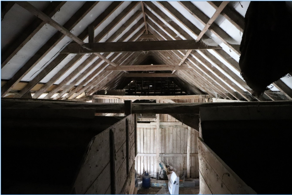
Figure 12. The roof of the main barn, looking west, showing the wholesale replacement of the roof structure in modern materials.
