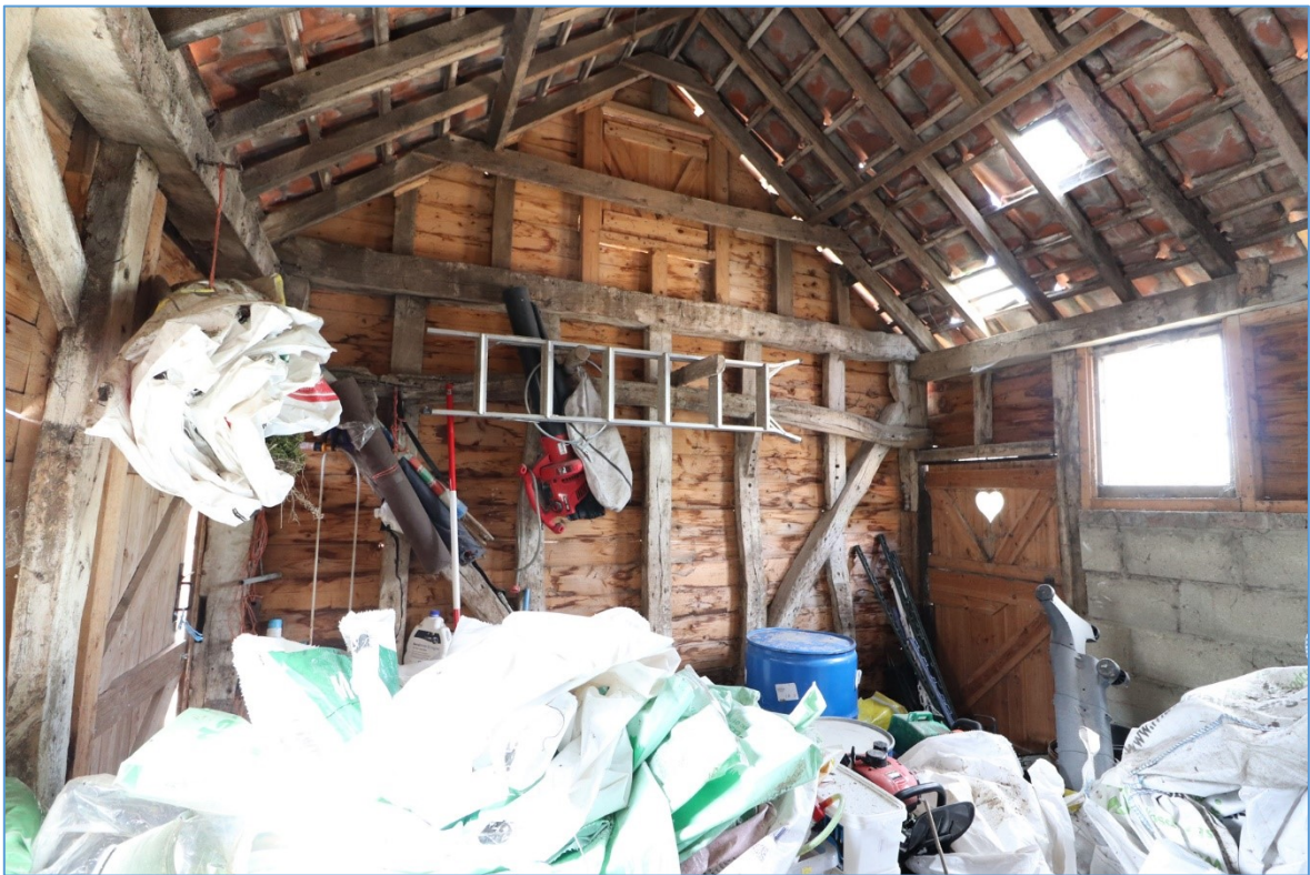
Figure 54. The northern wall of the smaller barn, looking north, showing the surviving timber framing.
