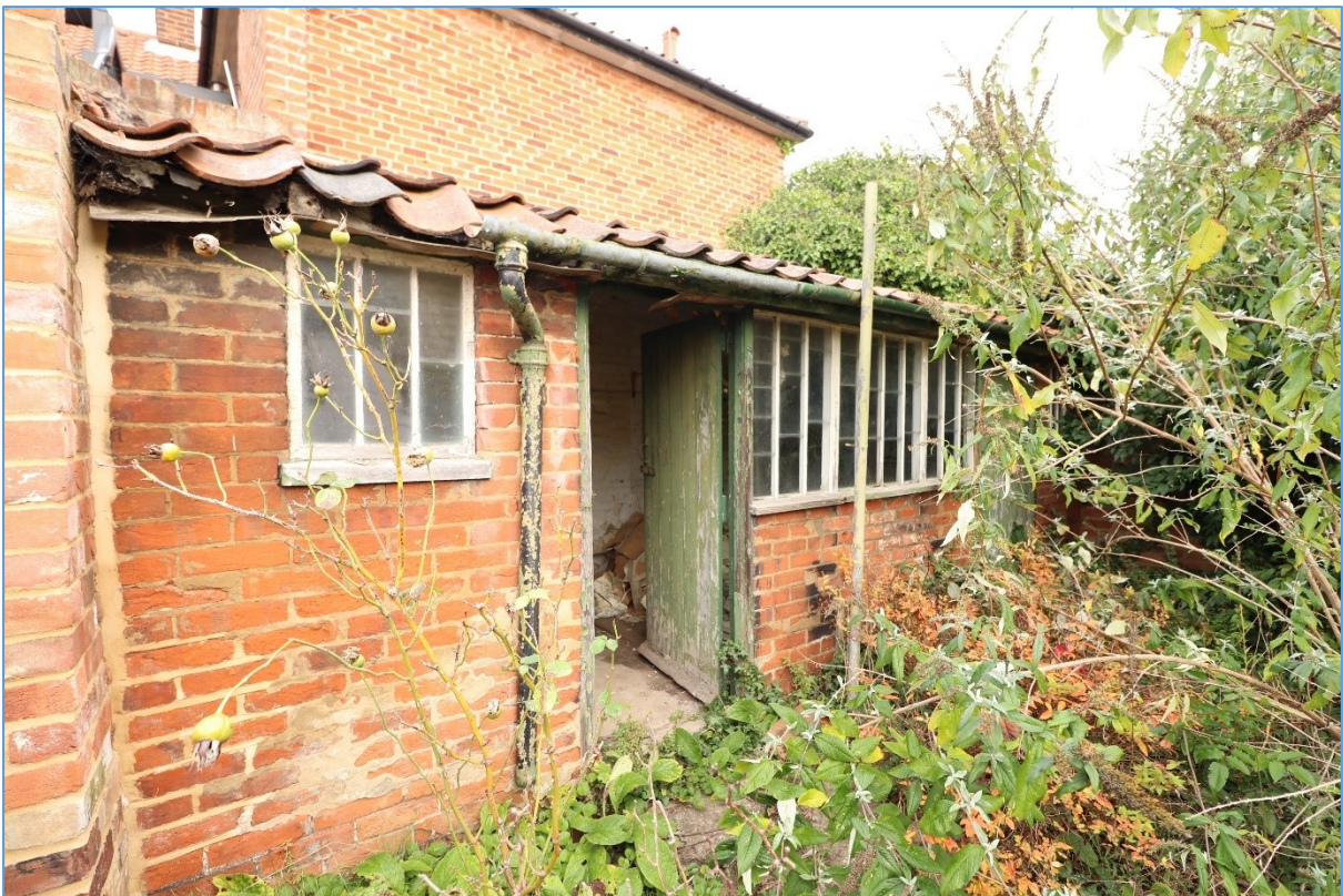
Plate 26. The exterior of the full-width outbuilding, looking north-east, showing both doors and glazed front.
