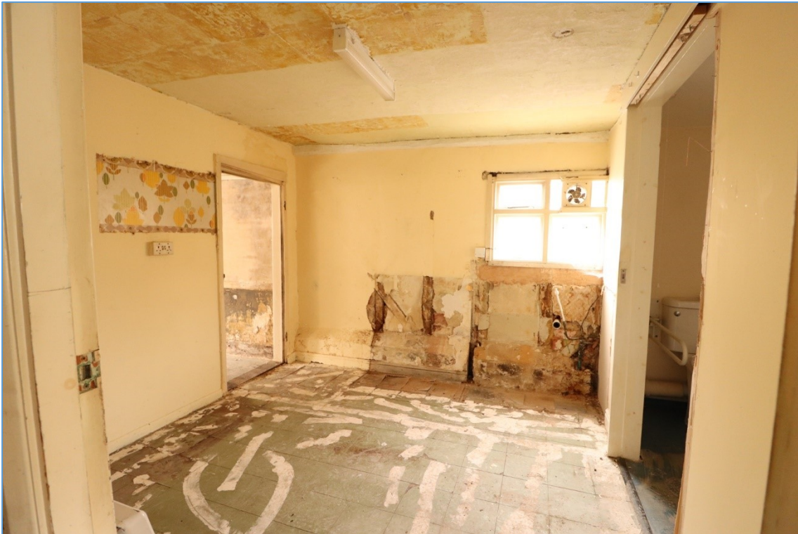
Plate 10. The north-western former kitchen, looking west, showing exposed timber framing and entrance to the modern bathroom to the north.
