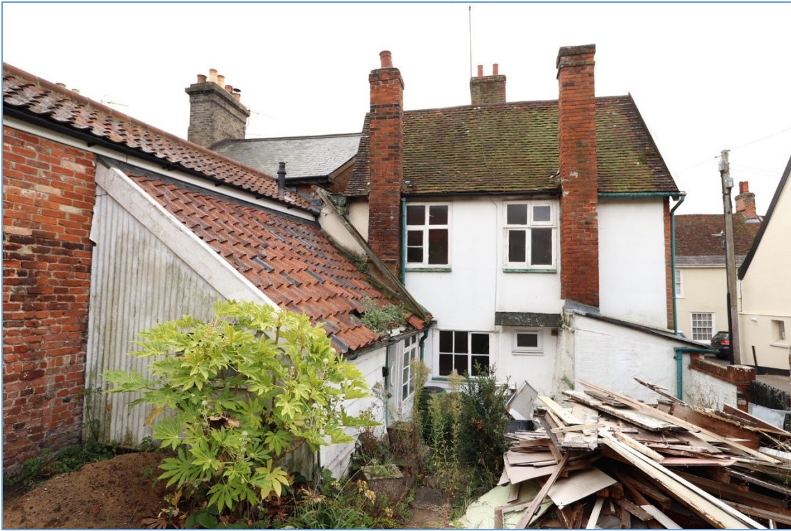
Plate 4. The property from the north, showing the rear elevation, with chimneystacks and extensions fronting onto a small yard.
