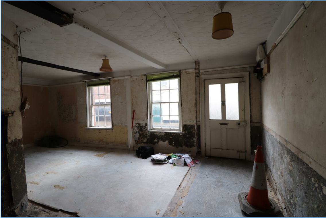
Plate 6. The ground-floor front room, looking south, showing front door, and wall and floor scars of former partition walls.
