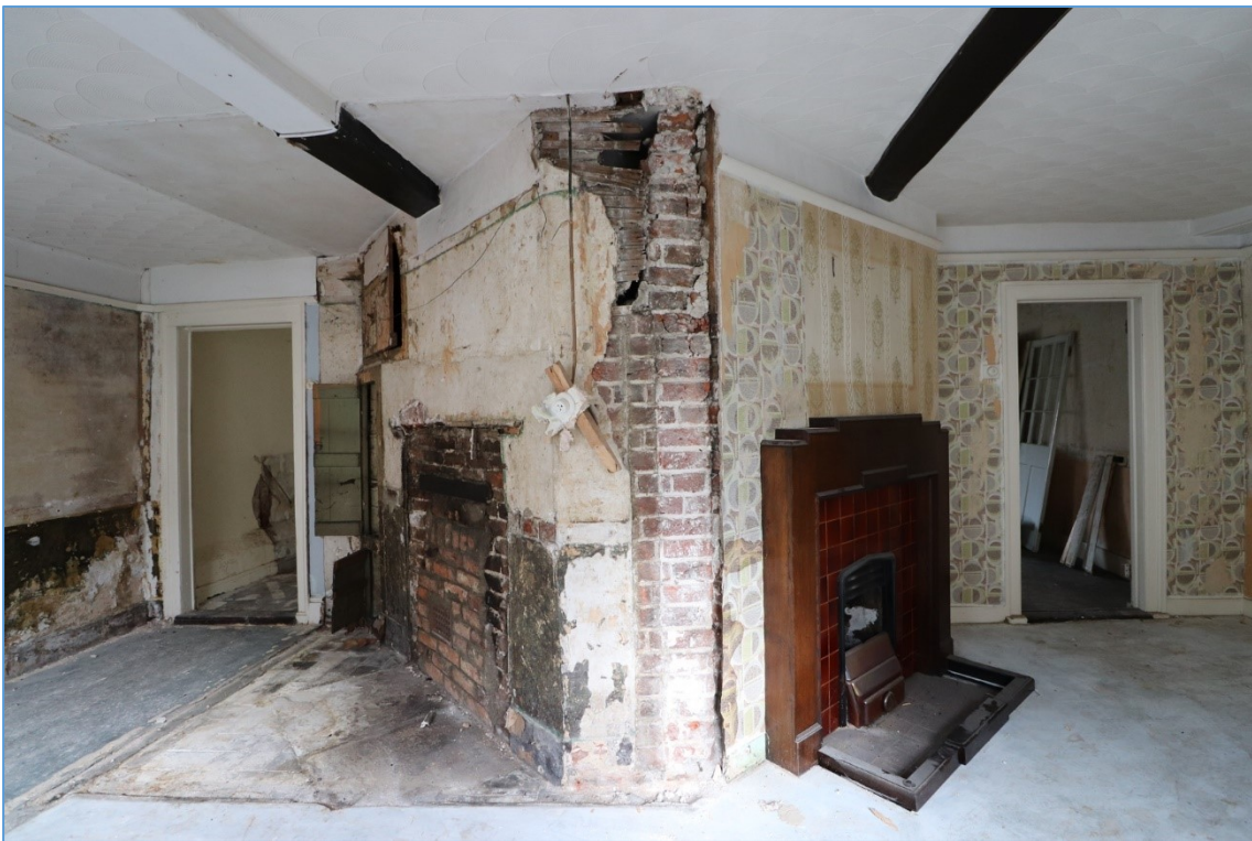
Plate 7. The central chimney stack, looking north along the line of the original partition wall, showing the blocked western fireplace and the open eastern fireplace.
