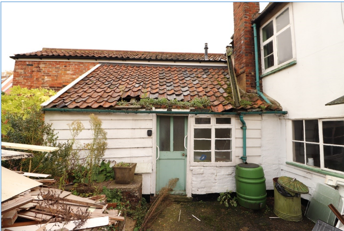
Plate 5. The western façade of the north-eastern extension, showing weatherboard construction and dilapidated condition of the roof.
