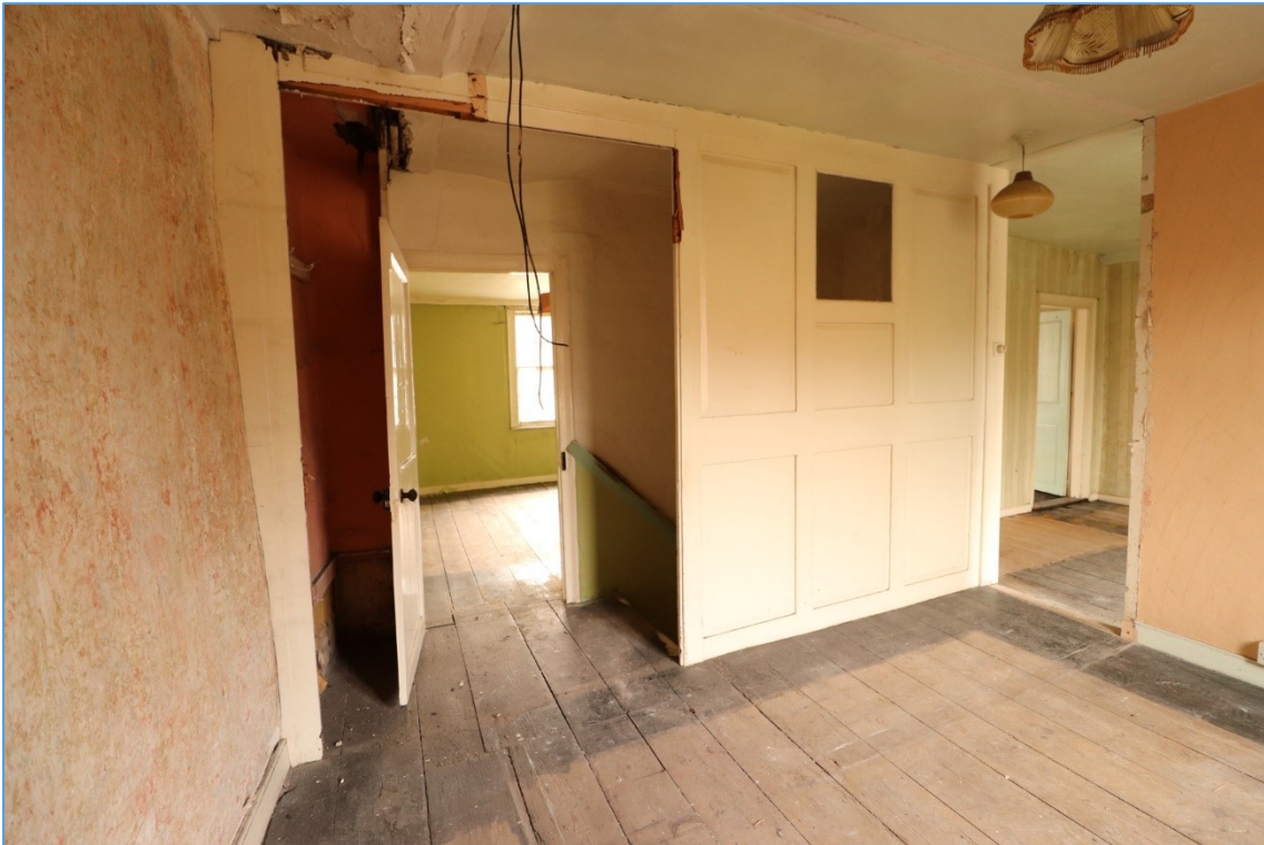
Plate 18. View of the landing, looking south, showing the scars of former partitions and linking doorway.
