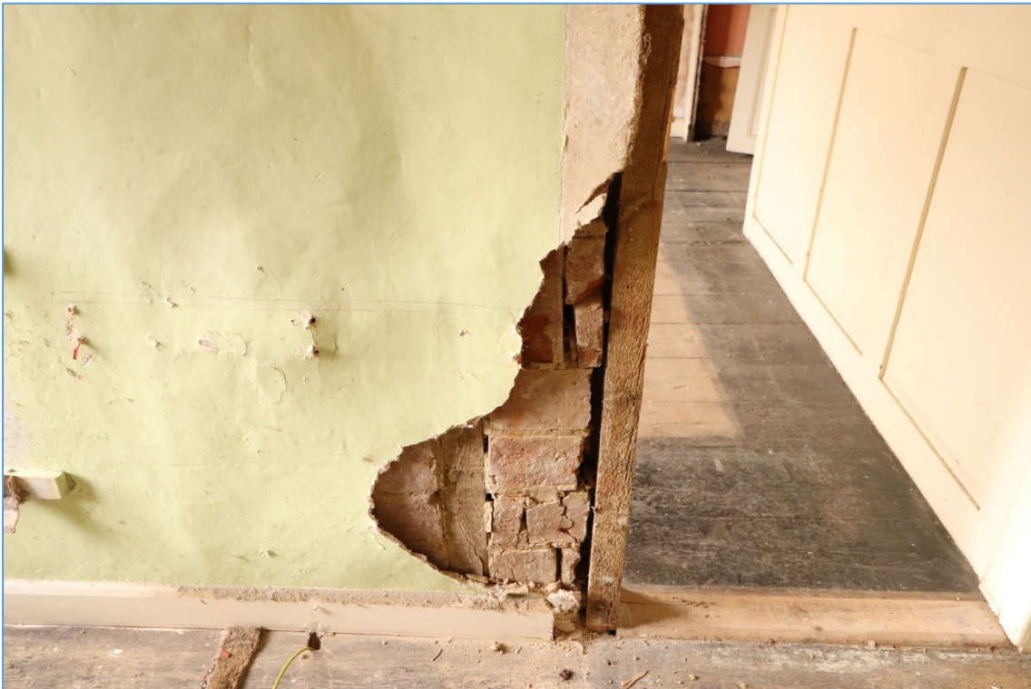
Plate 21. Detail of the construction of the partition wall between the properties, looking east.
