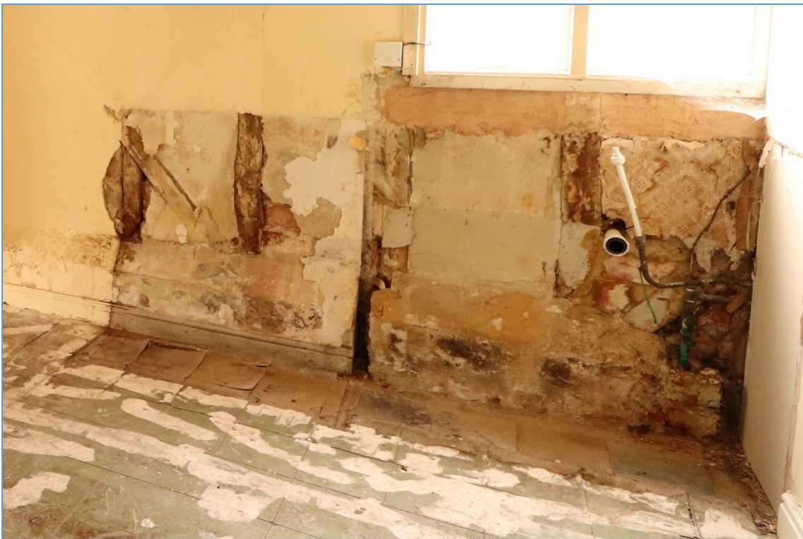
Plate 11. Detail of the exposed timber framing in the western gable wall of the former kitchen.
