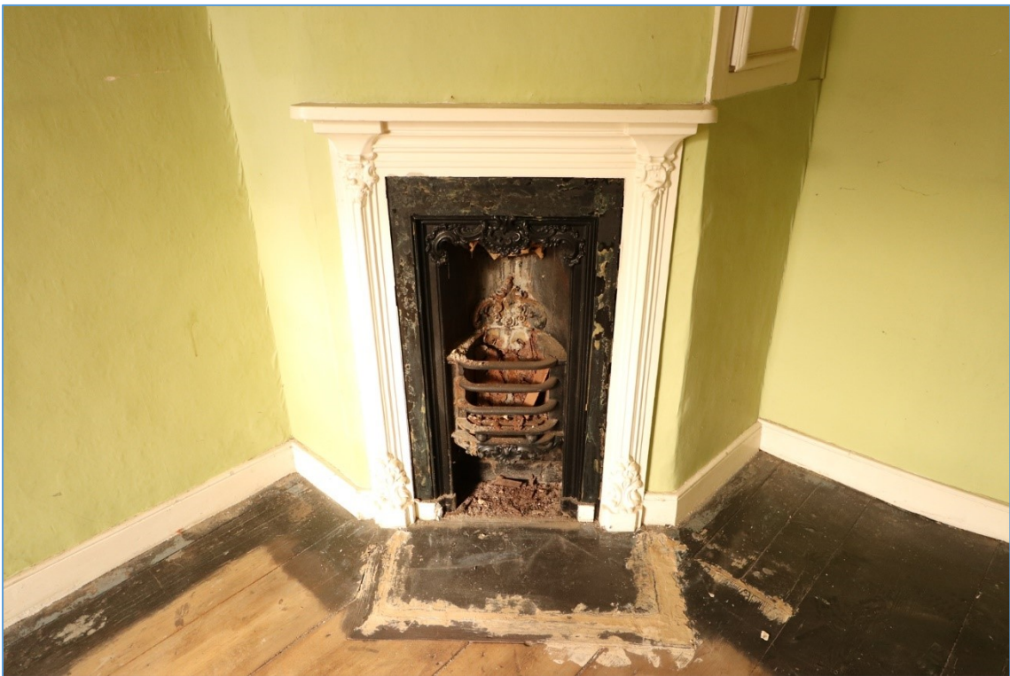
Plate 25. Detail of extant ornate fireplace in the south-eastern first-floor bedroom, looking north-west.
