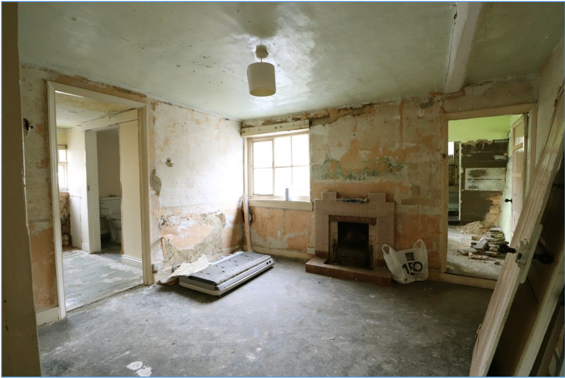
Plate 12. The north-eastern former dining room, showing extant fireplace and doorway to the extension.
