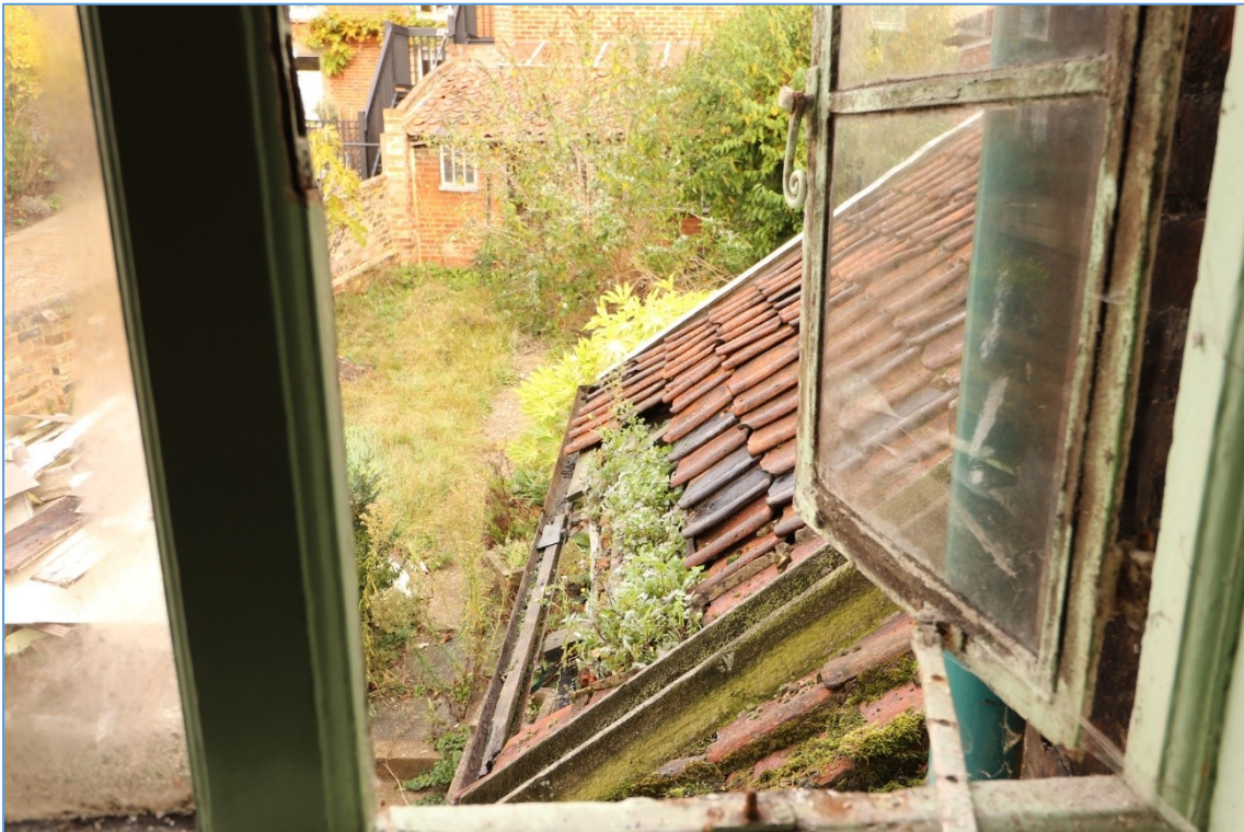
Plate 19. View from the rear bedroom window across the roof of the north-eastern extension, with outbuilding beyond.
