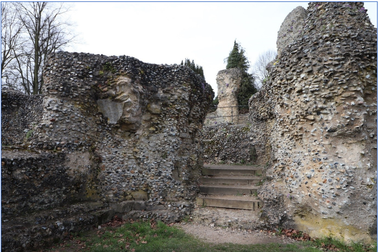
Figure 97: View of the surviving staircase leading from the south transept to the crypt, looking west.
