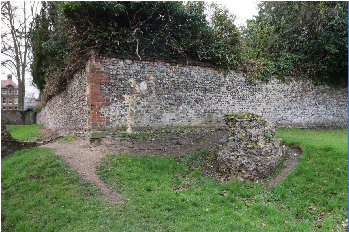
Figure 107: The eroding foundations of the north-eastern corner of the Deanery's garden wall, which was clearly constructed on top of the post-Dissolution rubble layer.
