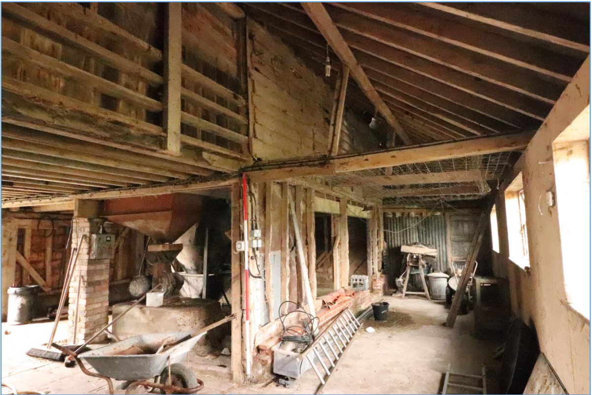
Plate 26. Interior of the northern bay of Building B and its eastern aisle, looking north.
