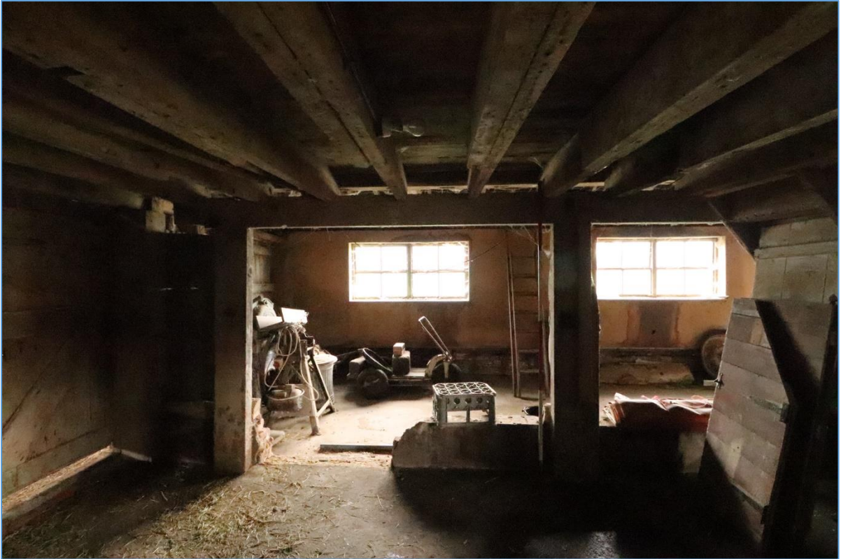
Plate 27. Interior of the northern bay of Building B and its eastern aisle, looking east.
