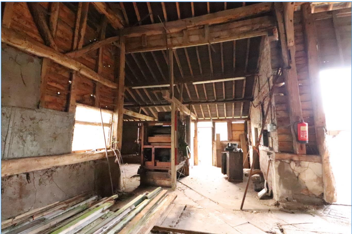
Plate 10. The interior of the southern bay of Building A, looking west into the south-western lean-to.
