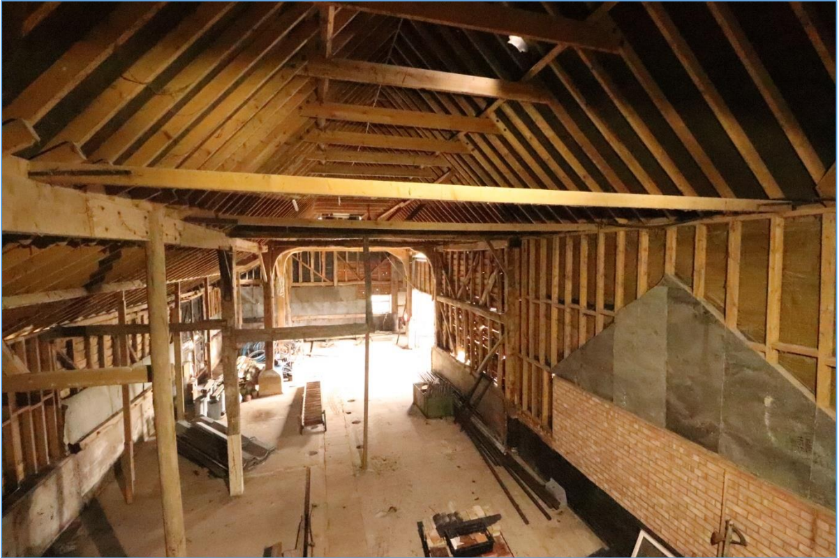
Plate 51. Interior of Building E, looking south from the first-floor of Building B.
