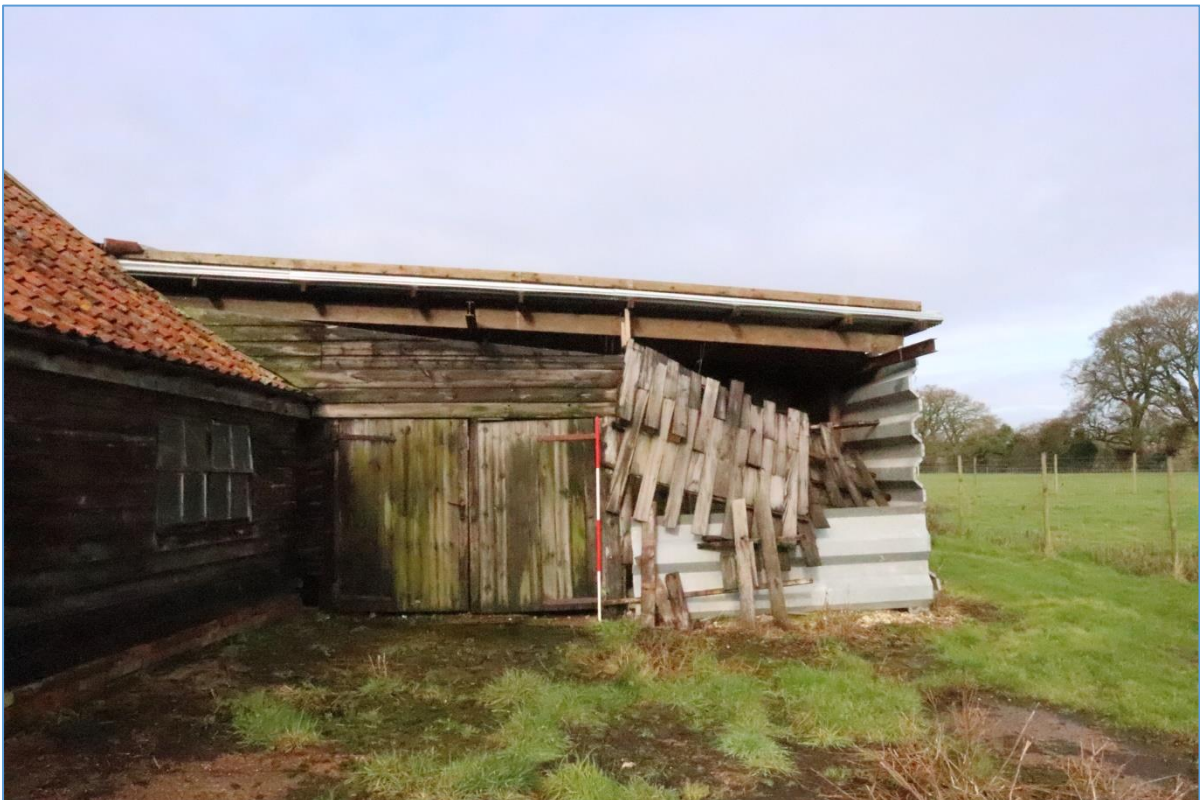
Plate 22. The southern elevation of the lean-to structure north of Building B, looking north.
