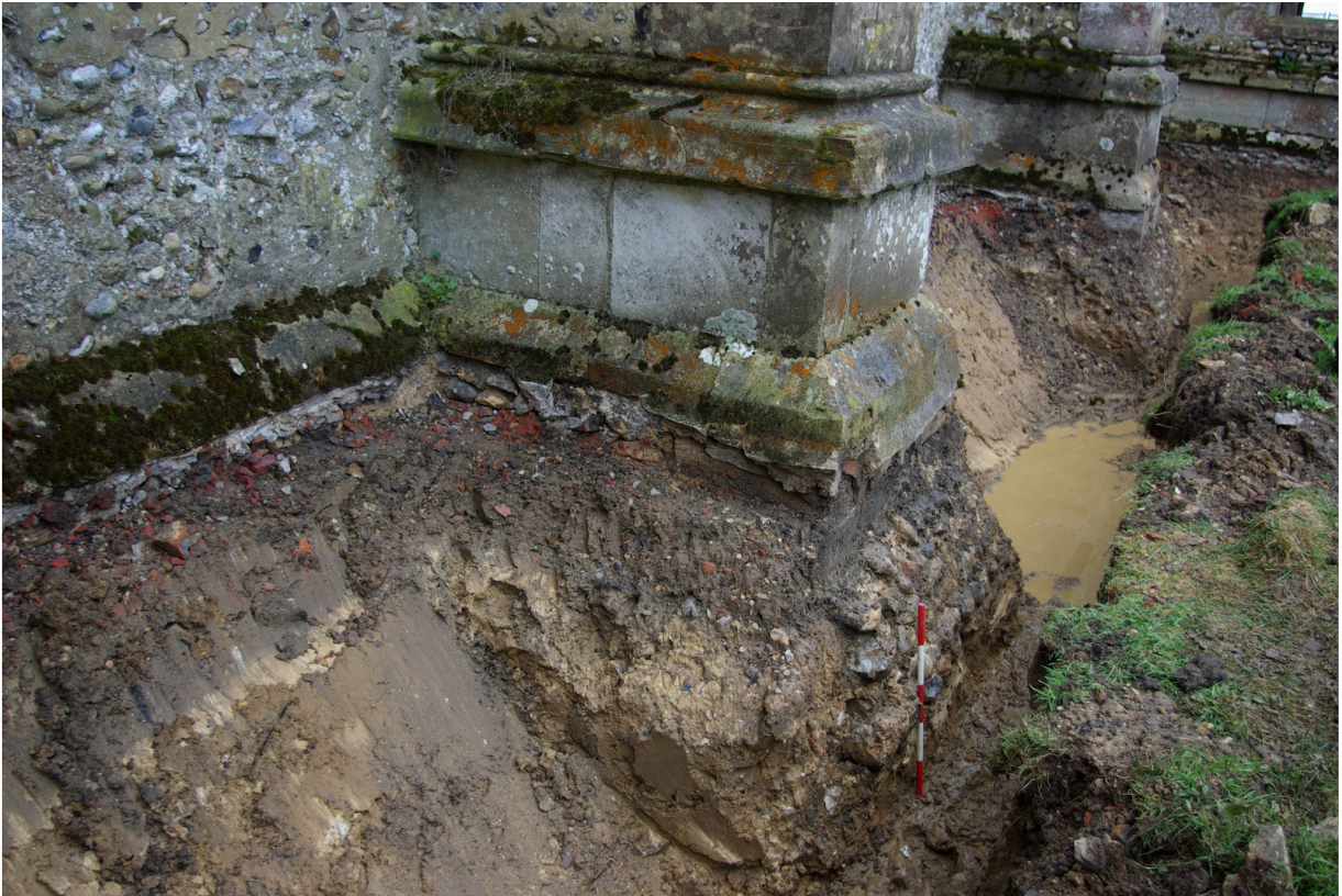
Plate 5: N nave central buttress with footing 5 and cream clay, looking SW, 0.5m scale
