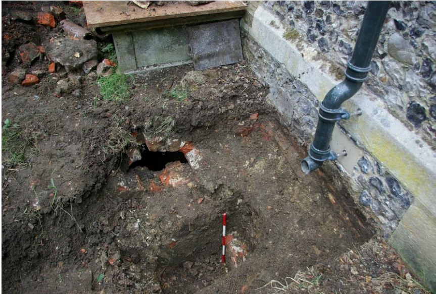
Plate 4: Gully trench 4 with brick feature 15 (0.5m scale) and showing damage to vaulted structure 16, looking SSW
