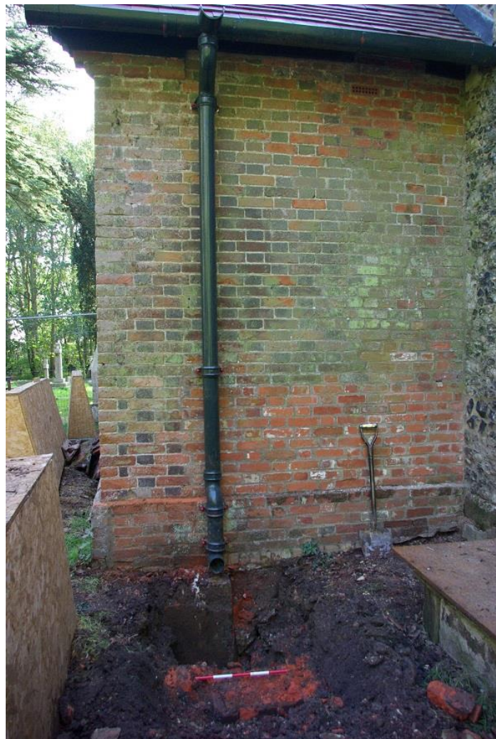
Plate 5: Gully trench 5 with brick wall 6 (0.50m scale), looking S and new brickwork in chancel wall visible
