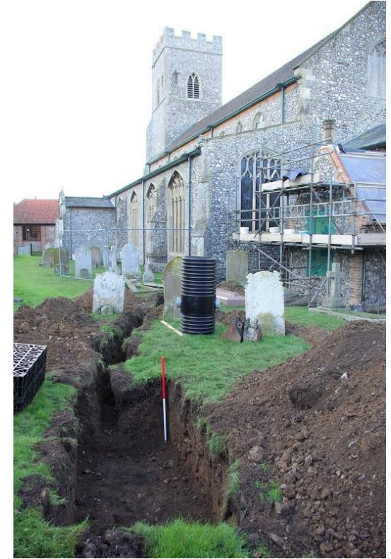
Plate 16: Trench [36] and drains S of church, south porch visible, looking WNW, 1m scale
