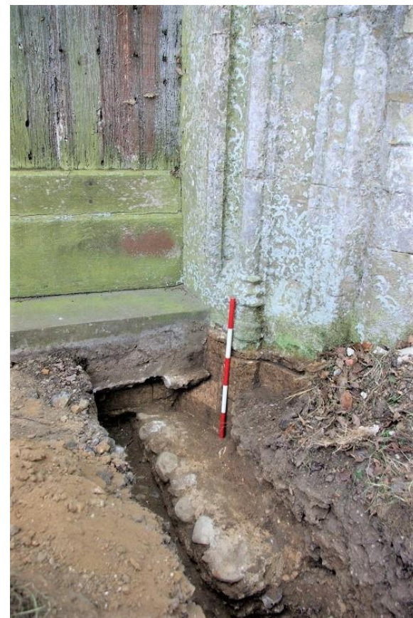
Plate 2: Trench 1; footing [6] with base of door jamb exposed, looking ESE, 0.5m scale
